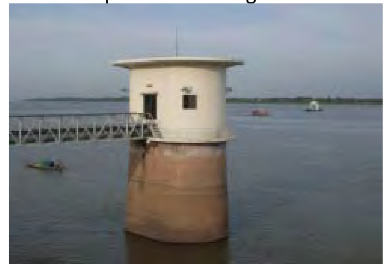
Sumpwell in Mekong River
