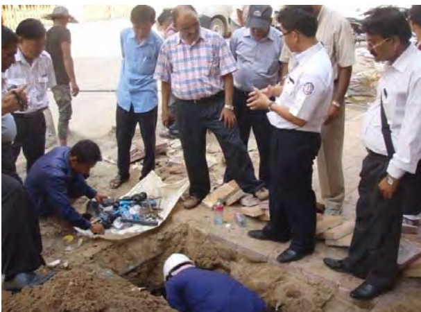
Photo-4 Third country Training in PPWSA in Cambodia House connection construction site Connecting from distribution pipe
