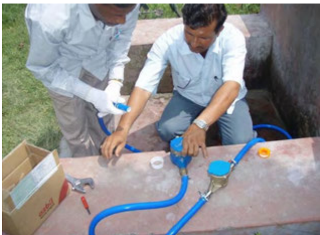
Examination of instrumental error with reference (standard) water meter for Gauradaha WUSC's water meter
