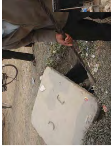
Gate valve chamber
