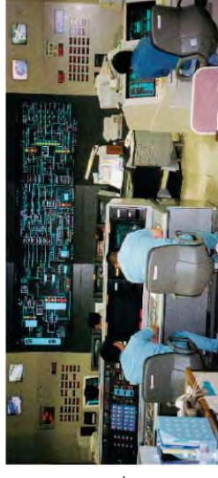
Sample of centralized computer control system, Tokyo Metropolitan waterworks
