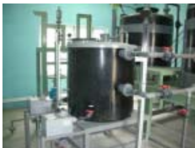
Chlorine facility at Gauradaha
