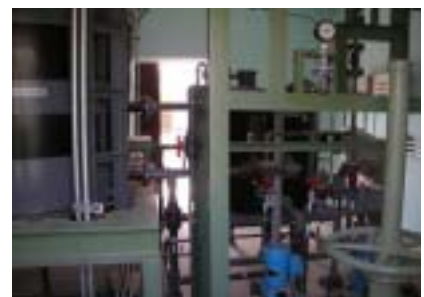
Chlorine facility at Mangadh
