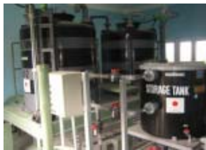
Chlorine facility at Dhulabari
