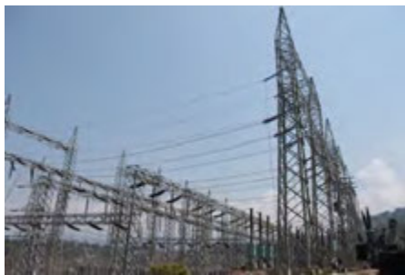
(a) Tsirang substation
