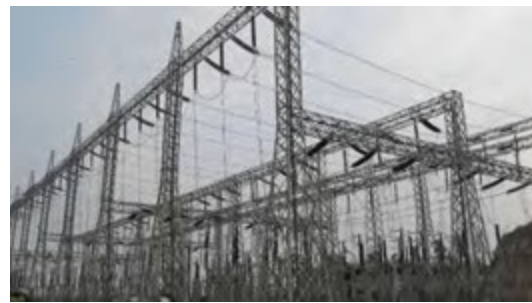
(b) Jigmeling substation
