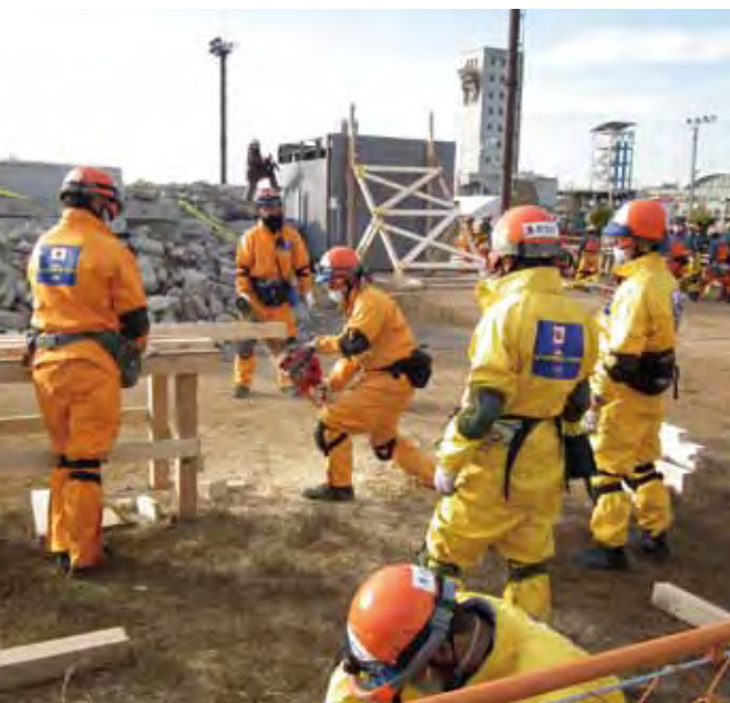
In accordance with international guidelines, Japan Disaster Relief Team maintains preparation and organization to execute their full capacity at oversea search and rescue mission. (Photograph is scene from general training at Nov. 2012)
