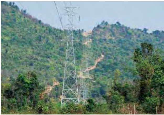
This transmission line of about 40km goes from the Paksan substation and over the Pakkading Pass.
