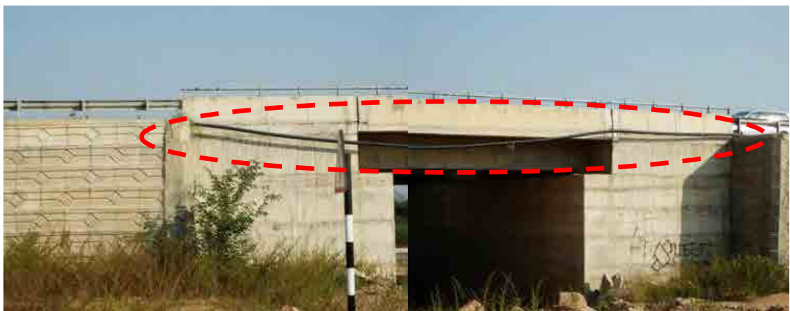
Hanging duct not fixed to parapet
