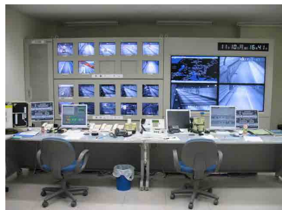
Photo 5.1: Example of Traffic Control Centre
