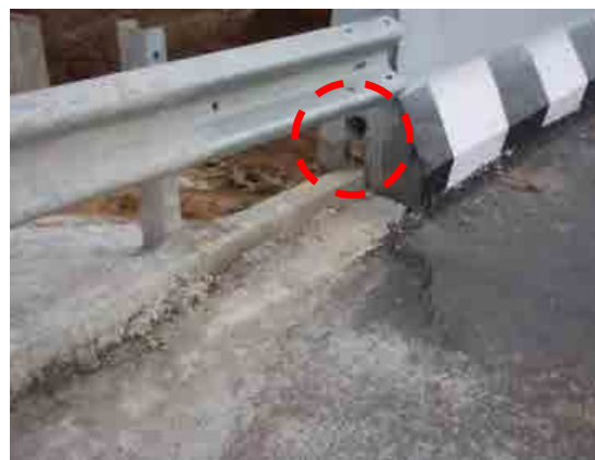
Duct not connected to underground section and
