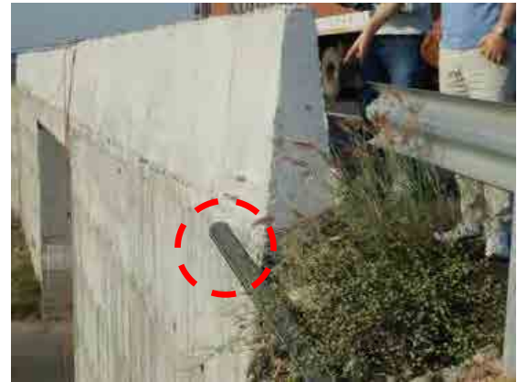
Duct not properly installed
