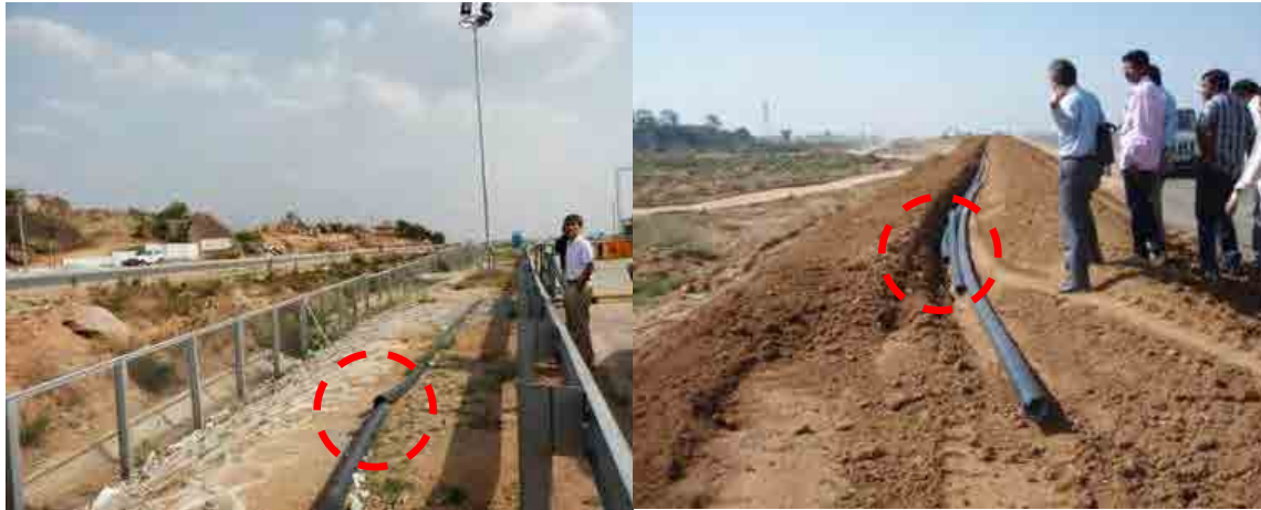
Duct not buried and probably not connected
