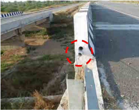
Ducts not connected to underground section
