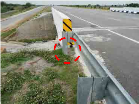
Duct not connected to underground section and clogged duct (lower side)
