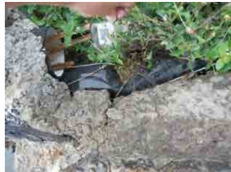
Damaged or disconnect ducts exposed on the ground
