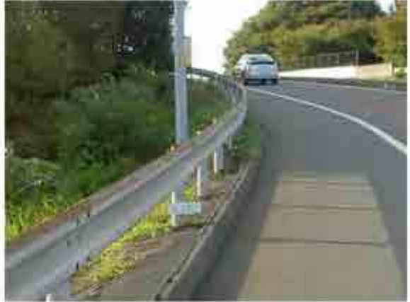
Stick type to guardrail pole
