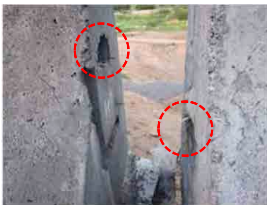
Ducts at different level and duct half covered with
