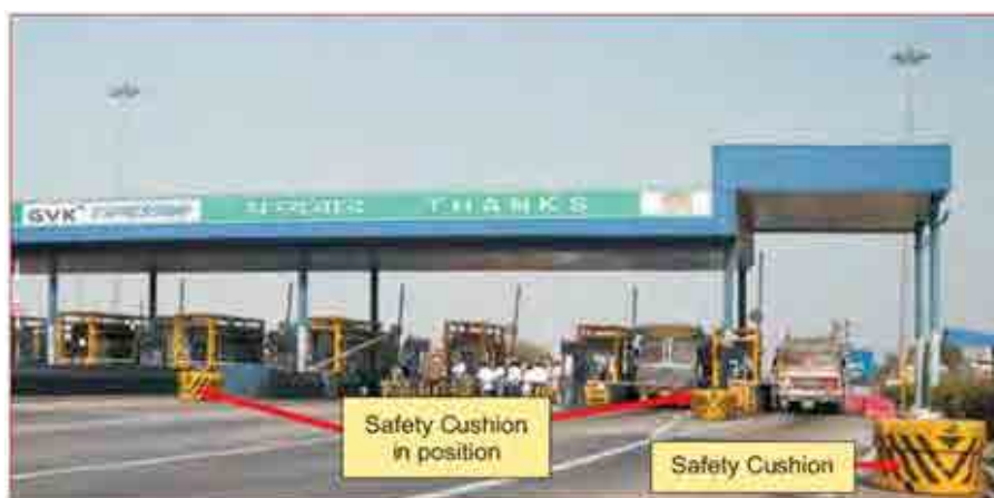
ORR will not require installation of safety cushions at the ends of raised toll booths as shown in the photograph above
