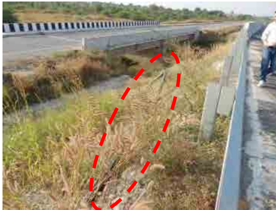
Duct not properly installed
