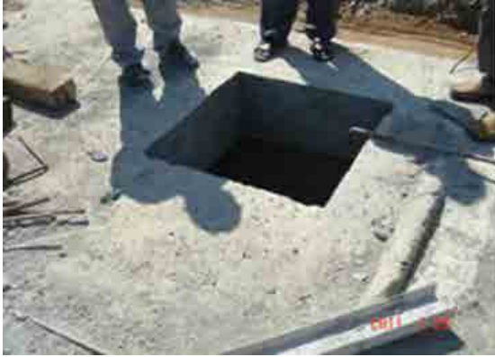
Opening of 80cm x 80cm too small for stair
