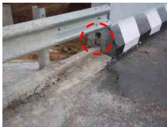
Duct not connected to underground section and clogged duct (lower side)
