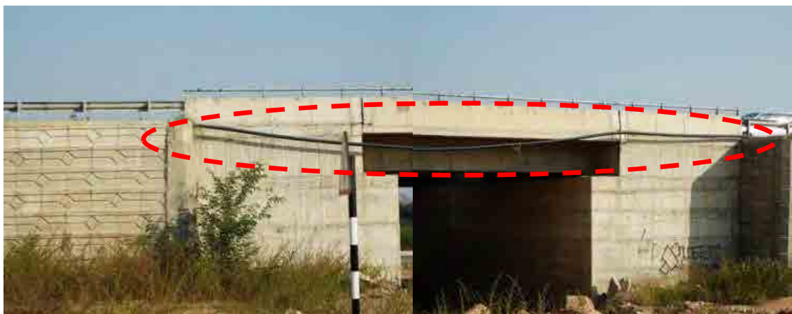
Hanging duct not fixed to parapet
