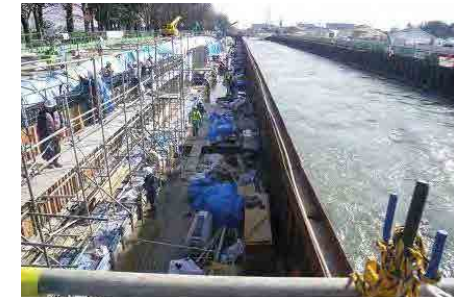
Construction with a large number of workers (maximum number of workers per construction area: about 100) 14
