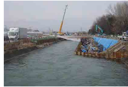
Difference of about 30 cm between the top of sheet piles, and the water surface
