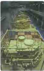
View of pump room
