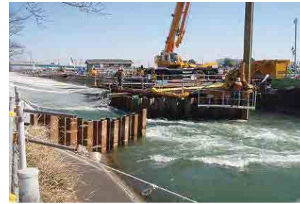
Construction work in the area with rapid water flows (flow rate of about 2 to 3 m/s)
