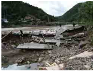
Levee breach site (provided by Kobe Shimbun)
