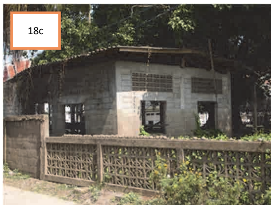
Figure F18 Comparison of damages between two-story houses in (a) and (b), which have different style of the lower story, and one-story house in (c)
