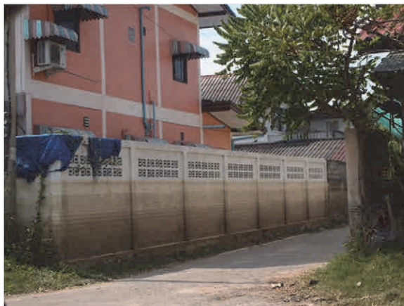
Figure F14 The flood height is around 2-m from existing road in in Kung Samphao Sub-district, Manorom District, Chai Nat Province.
