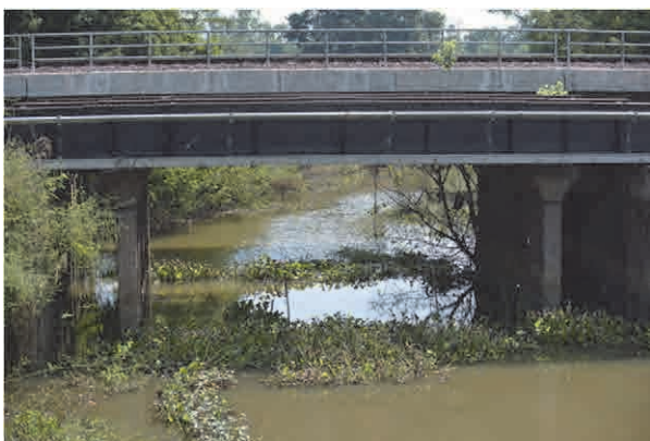
Figure F5 The piers of railway bridge, which is one obstacle for water draining (Ayutthaya Province).
