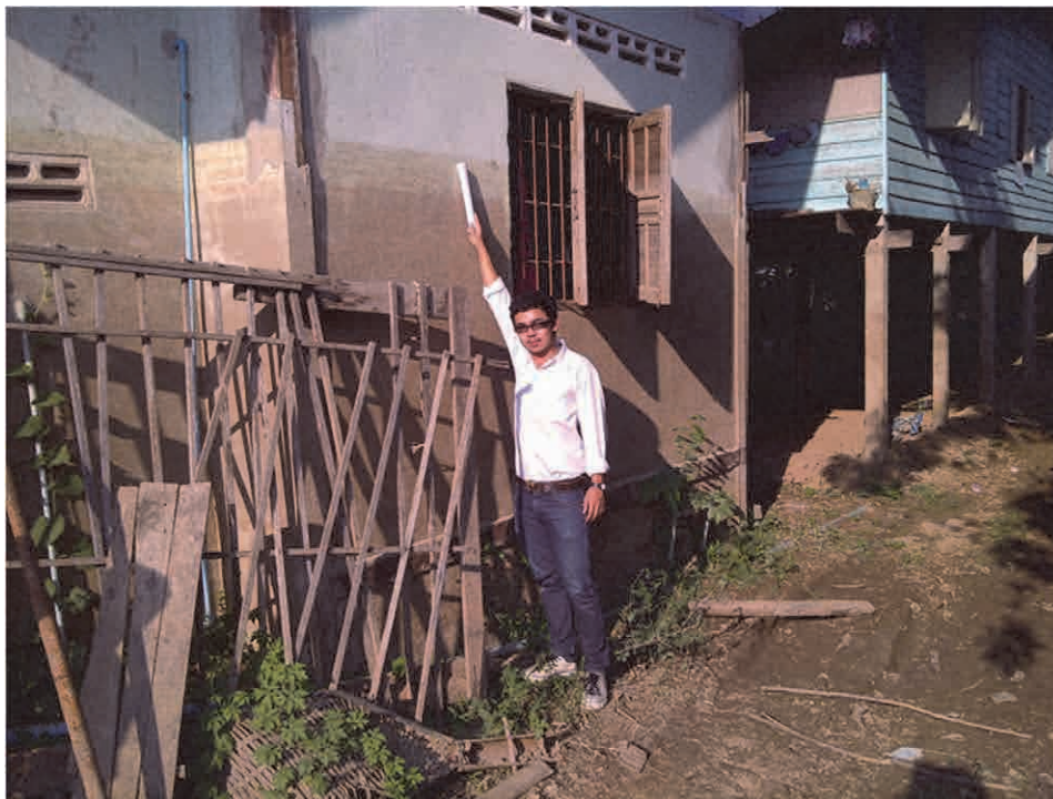
Figure F17 Over 2-m flood level in Khok Kateam Sub-district, Muang District, Lopburi Province
