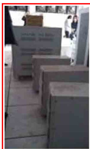
UPS Room (1st Floor)
