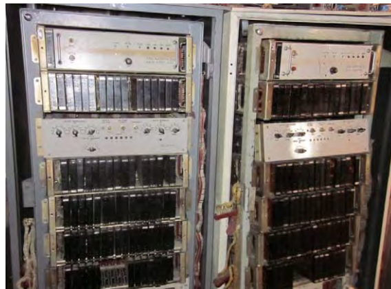
Picture 9.1-1 Defunct Local Controller Retrieved from Intersection
