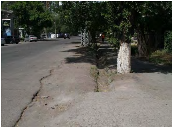
Picture 10.5-3 Deteriorated Road Shoulder Pavement
