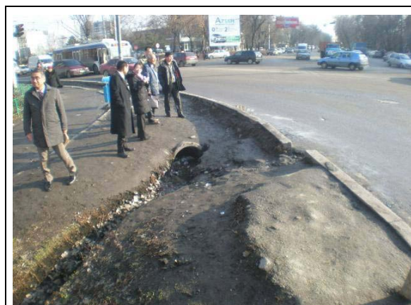
Deteriorated Drainage Facility & Discontinued Pedestrian Crossing
