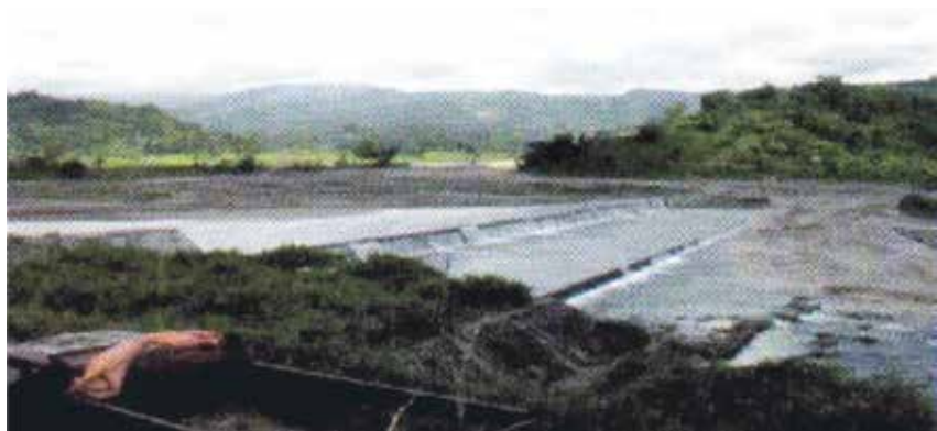
Figure 19: SP-5 after Mount Bawakaraeng landslide Source: BBWS Pompengan-Jeneberang
