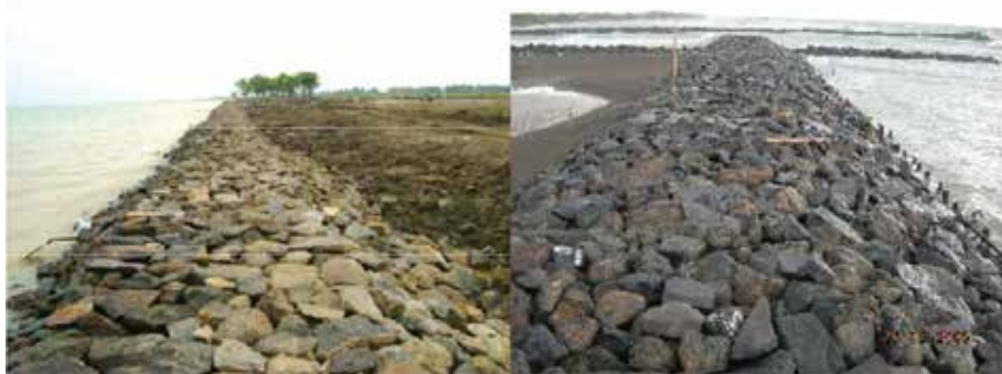
Figure 19: Management of abrasion in Indramayu Beach and PondokPutri Beach, Subang Regency
