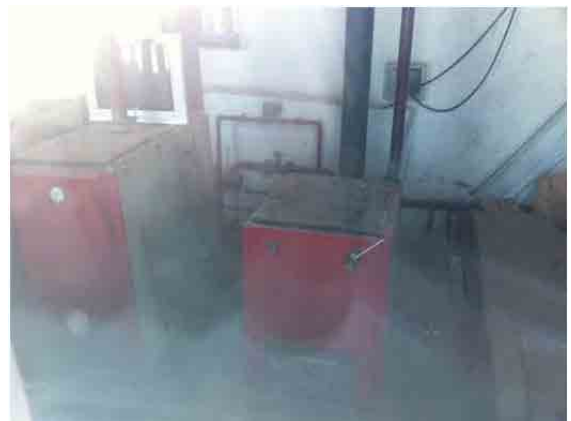
Individual heating system in kindergarten
