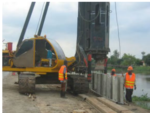
Flood wall is under construction on the southern bank of Phraya Banlue Canal (taken on Nov.17, 2012)
