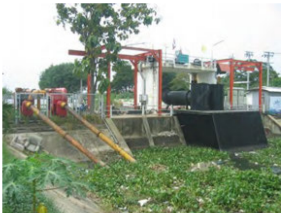
Bang Talat Regulator and Pump Station (RID Nonthaburi), two semi-permanent pumps (black ones) were urgently installed after the 2011 flood. (taken on Nov.16, 2012)
