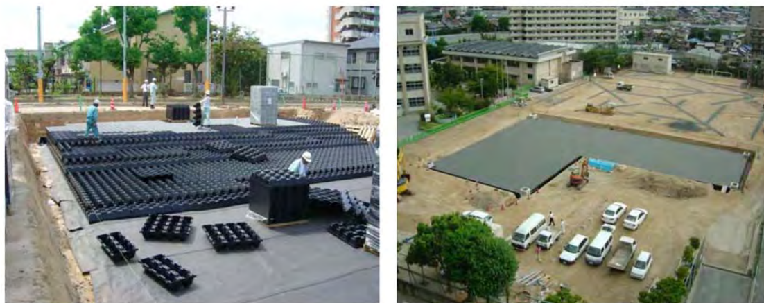
Figure 2.1-3 Examples of On-site Storage Facility using Plastic Material
