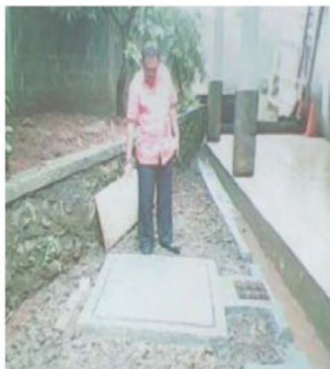
Infiltration Facility (Example in Bogor)
