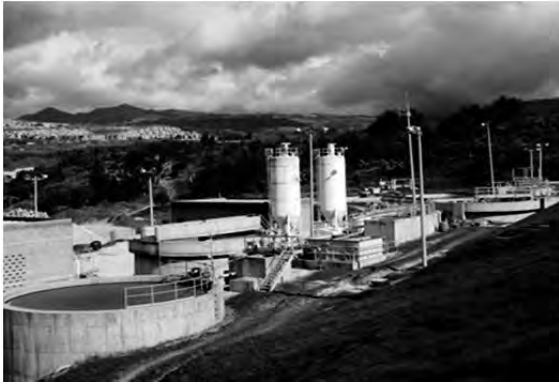
Treatment Plant for Percolated Liquids
