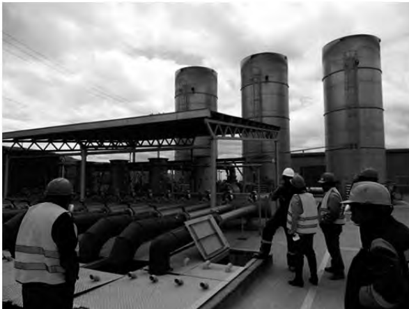
Biogas Management Plant
