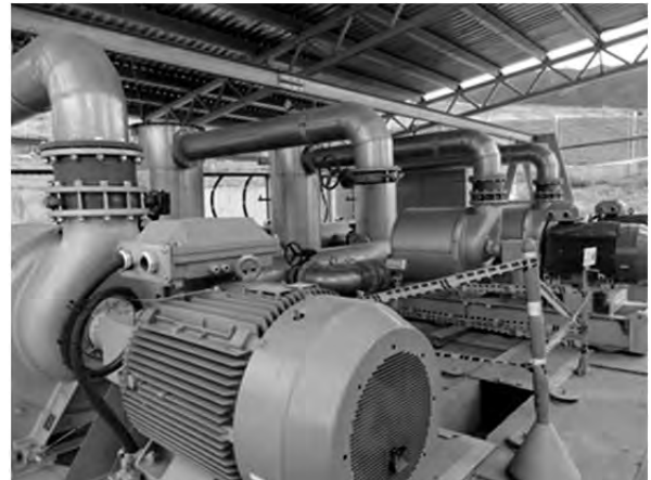
Biogas Management Plant
