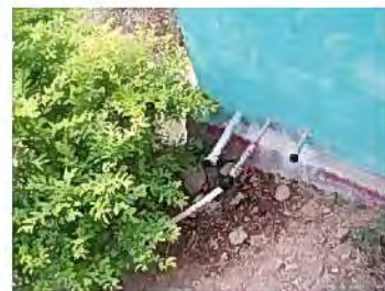
photo-10: additional outlet pipe
