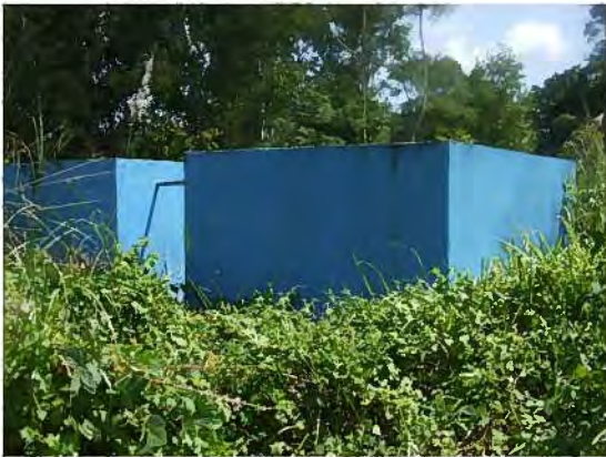
[Uma Boco-Fehuk Krin] – 3. Ground Storage Reservoir No.1 to the Town(20m 3 x 2 basins)
