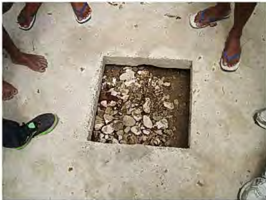
photo-3: the Intake facilities filled with sand and gravel
