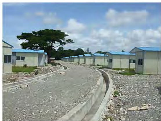
[Aubeon-Buburlaran] – 4. Earthworks not completed (Backfill observed insufficient)
