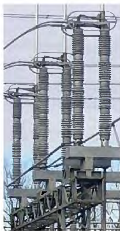
Post type insulators
