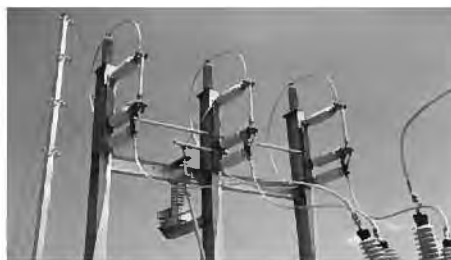
Vertically Mounted Vertical-Break Switch
