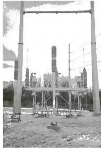
Station Post Insulator
