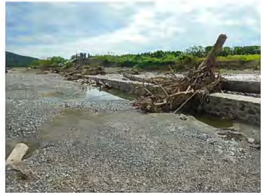
Washed Out of Revetment at End
