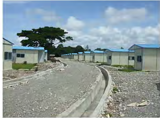
[Aubeon-Buburlaran] – 4. Ateru rai ladauk kompletu Earthworks not completed (Observa katak ateru lato) Backfill observed insufficient)
