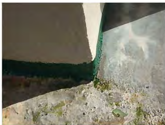
[F-FDTL] – 1. Hafoun hikas konstrusaun reservador bee suli liu ba kraik (Leaks from the Bottom of the Reservoir newly Constructed)
