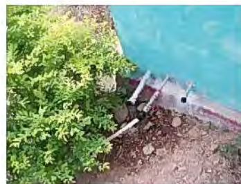
photo-10: additional outlet pipe
