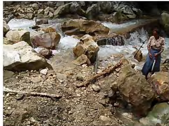
photo-3: the Transmission pipe crossing a fast-flowing stream
