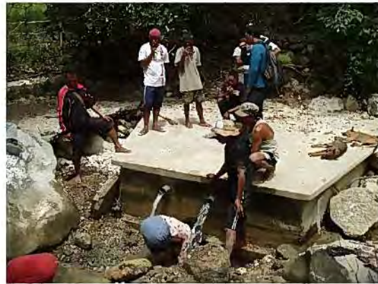
photo-2: the Intake facilities
