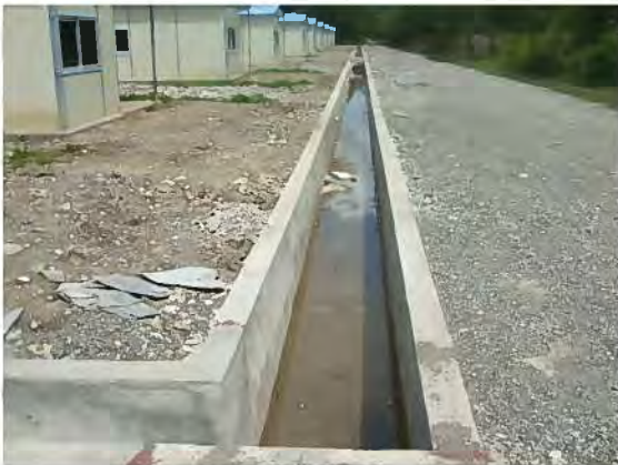
[Aubeon-Buburlaran] – 1. Stagnant Rain Water in Drainage Channel (Immediate repair ordered by ADN Engineer)
