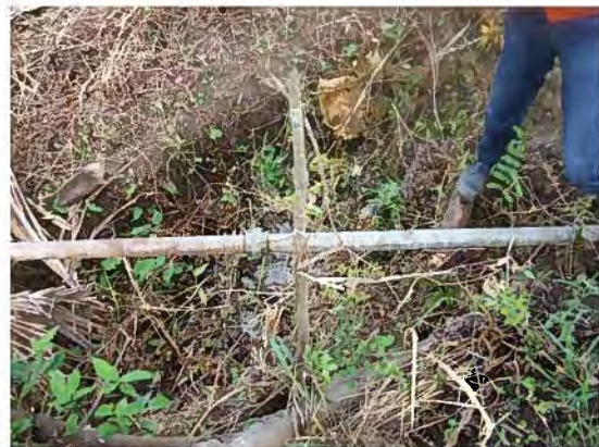
[F-FDTL] – 4. Existing Raw Water Transmission to F-FDTL (4km x 3" in diameter, GSP)
