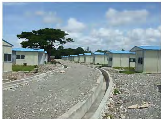
[Aubeon-Buburlaran] – 4. Earthworks not completed (Backfill observed insufficient)
