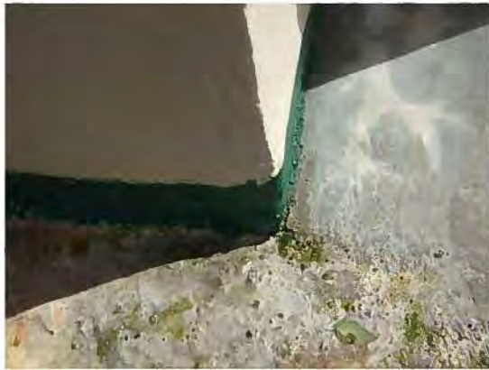
[F-FDTL] – 1. Leaks from the Bottom of the Reservoir newly Constructed
