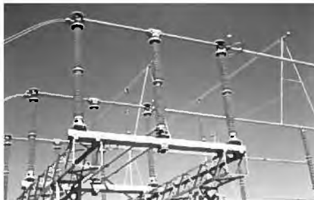
Horizontally Mounted Double-Break Switch
