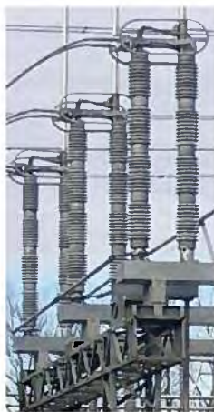
Post type insulators
