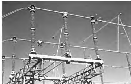
Horizontally Mounted Double-Break Switch.
