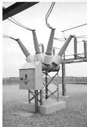
“Dead Tank” Breaker
