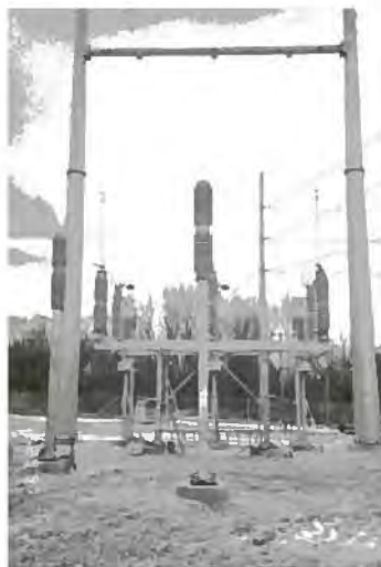
Station Post Insulator
