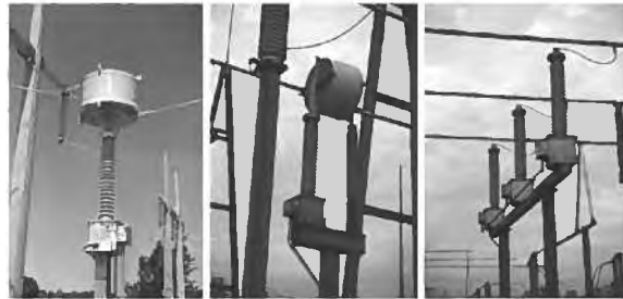
Coupling Capacitor Voltage Transformers With and Without Wave Trap
