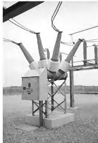
“Dead Tank” Breaker
