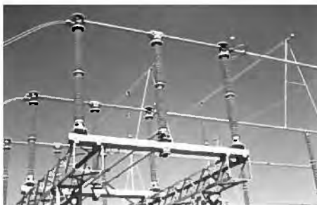
Horizontally Mounted Double-Break Switch
