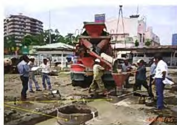
Stand Pipe 1 Protection Casing
