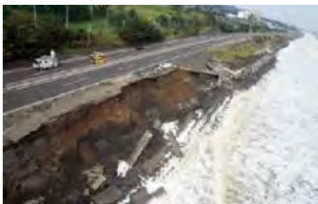
Figure: Seawall damaged by a typhoon
