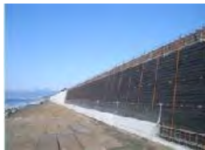
Figure: Restoration of seawall damaged by a typhoon using reinforced retaining wall
