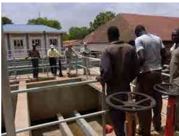
Water sampling for backwashing of filtration basins
