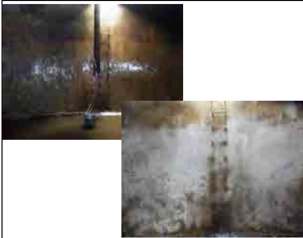
Cleaning activities for the clear water tank Before and after the tank inside
