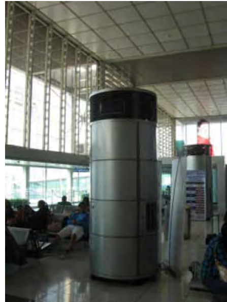
Central air-conditioning system in Ninoy Aquino International Airport, Terminal 2
