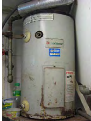
Photo. Conventional Electric Water Heater Installed in the Ninoy Aquino International Airport, Terminal 2
