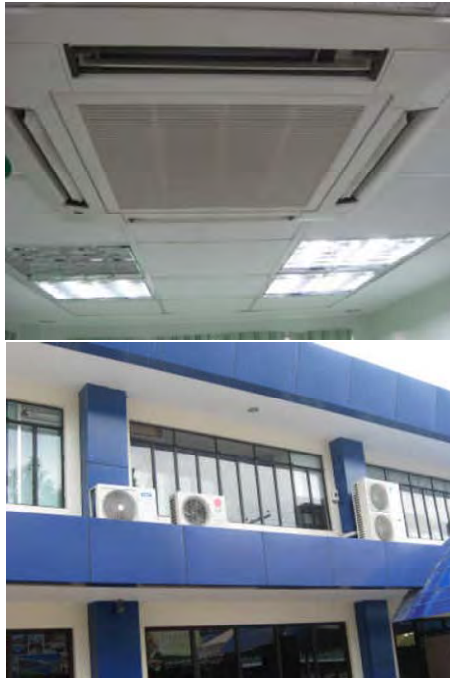
Air conditioning system in Tagbilaran Airport (top: indoor unit, bottom: outdoor unit)
