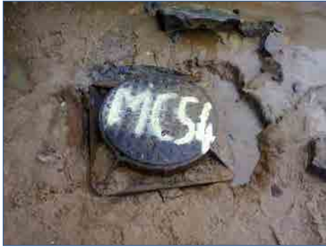
No concrete cover
