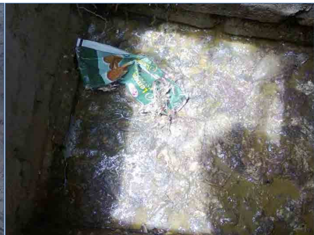
Poor workmanship causing subsurface infiltration
