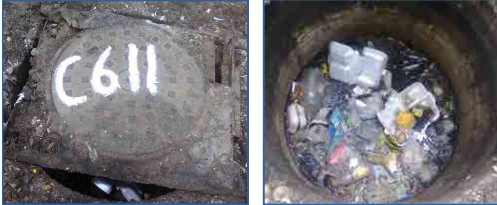
Photo 7.2.9 Manhole in a Public Area Used as Rubbish Dump
