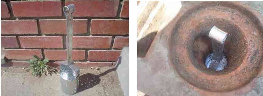
Photo 5.2.1 Sand and Grease Trap
