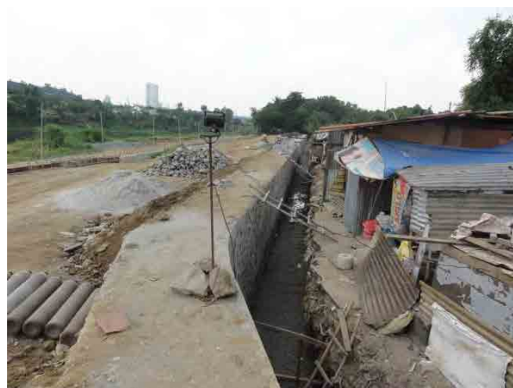
Parapet is being constructed in Santolan by Pasig City See Figure 3.20 for this position
