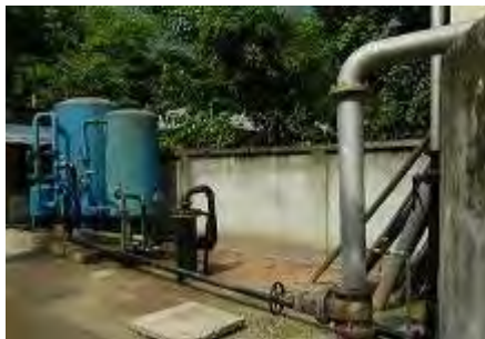
Groundwater Treatment Plant of BWSPP in Keraniganj, Dhaka Division
