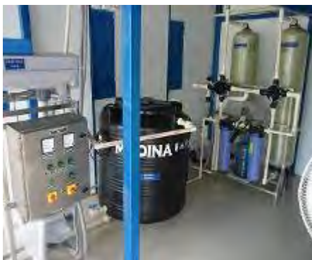
Water Treatment Equipment inside a WHC
