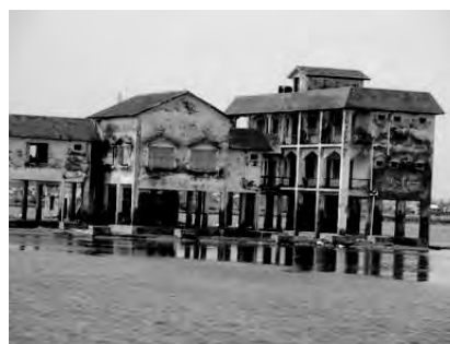
Salinity and brick structure
