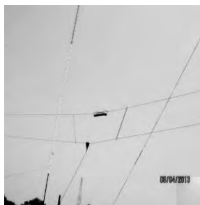
Wireless Antenna in DRRO office
