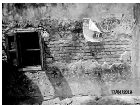
Damaged wall by saline water
