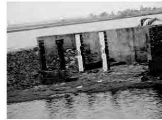
Salinity and brick structure
