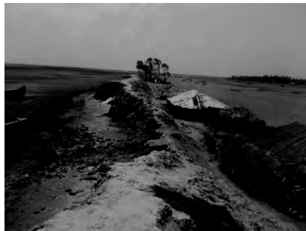
Picture: Damaged polder in Chhonua; there are 7-8 damaged sites along the polder.
