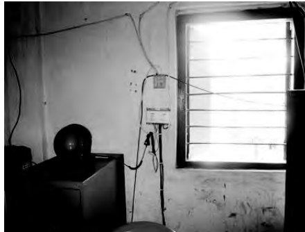
Terminal for solar system
