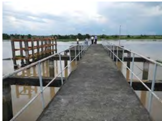
Hoa Phu Intake Pump N=3 (1)
