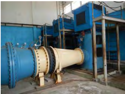
Sai Gon River Hoa Phu Intake
