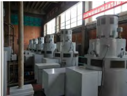
Dong Nai River Hoa An Intake
