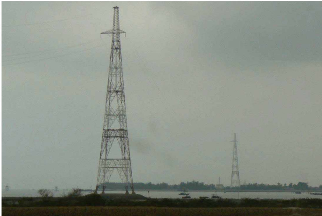
Photograph of high voltage towers and cables crossing the Channel. The photograph was taken from Cat Ba Island. Cat Hai side can be seen in the distance.
