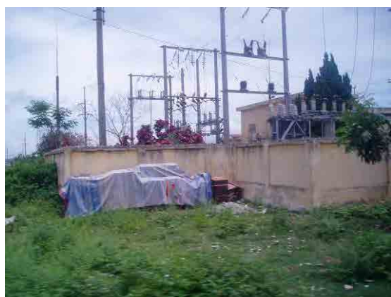
Photo 1 Old Substation in Cat Hai Island
