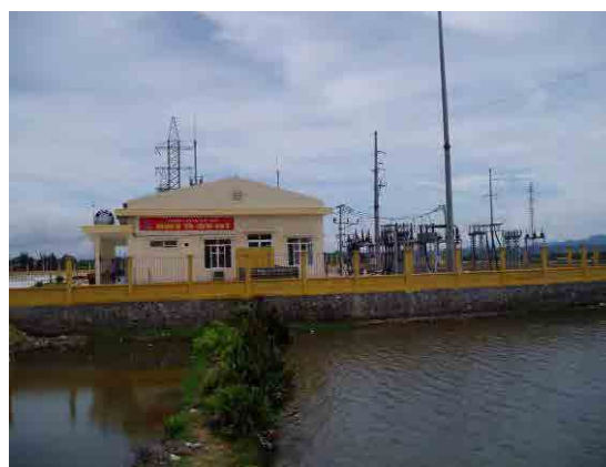
Photo 2 New Substation in Cat Hai Island
