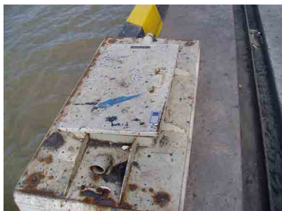
Photo 3 Utility Box (Water Supply)
