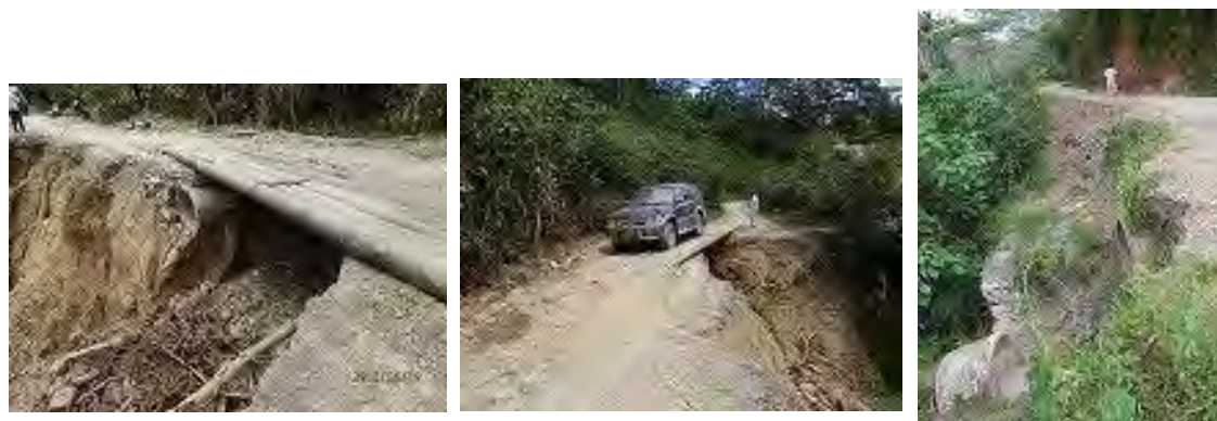
Photo 3.10 Road swept away due to culvert failure and pavement condition of Route A10
