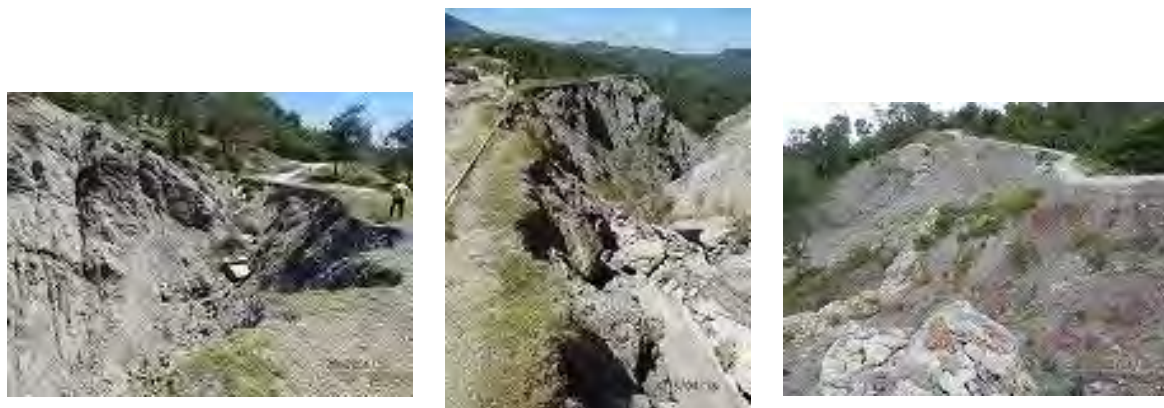
Photo 3.11 Large-scale collapse and pavement condition of Route A12
