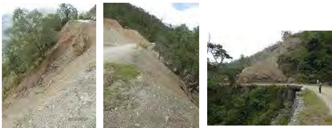
Photo 3.9 Large-scale collapse and pavement condition of Route A05
