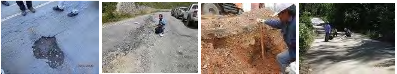
Photo 2.7 Examples of damage to the pavement in the section of Route A02 between 0 km and 79 km
