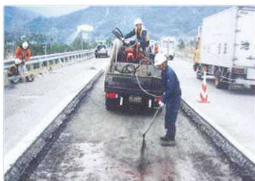
Laying a prime coat on a lower base course using an engine sprayer.
