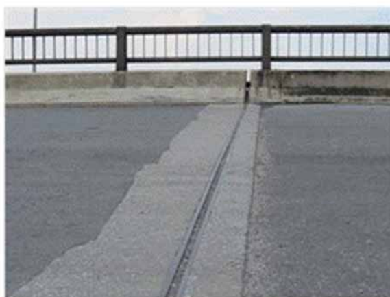
A bump at a bridge joint.
