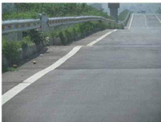
Deterioration of smoothness due to settlement in the front and rear of the structure
