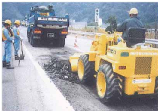
Demolishing an existing pavement and transporting the pavement waste using a shovel loader.
