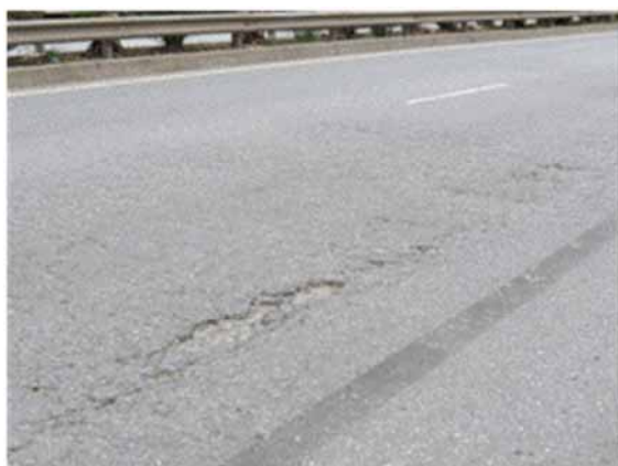
Deterioration of smoothness due to surface settlement with the development of cracking
