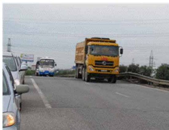
Deterioration of smoothness due to differential settlement near a transverse structure
