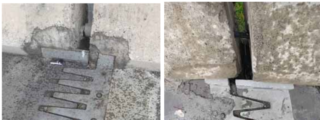
Figure 2.4-2 Inappropriate Water stop Works at Both Ends of Expansion Joint
