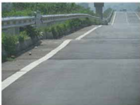
Deterioration of smoothness due to settlement in the front and rear of the structure
