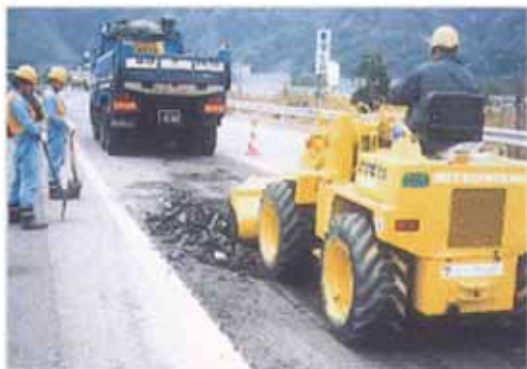
Demolishing an existing pavement and transporting the pavement waster using a shovel loader.
