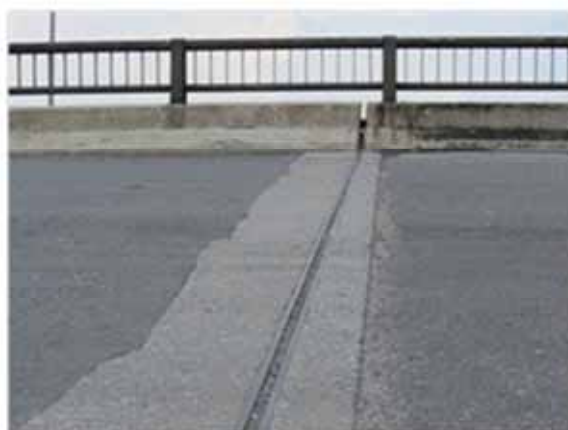
A bump at a bridge joint.
