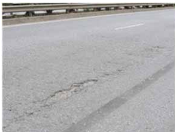
Deterioration of smoothness due to surface settlement with the development of cracking
