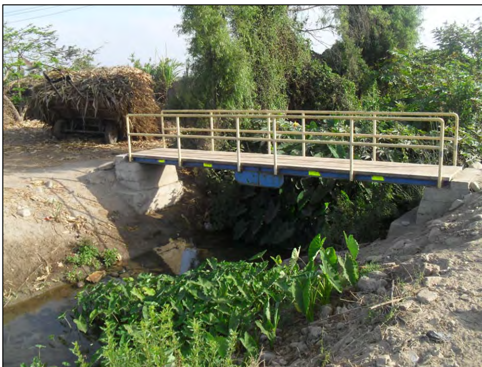
Figure 4.13 PACHACAMILLA Drainage (Ca-01)
