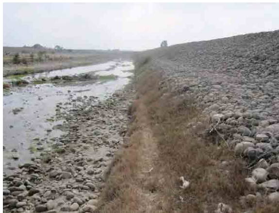
Figure 3.2 Dike Revetment by Mattress Basket in Chincha River
