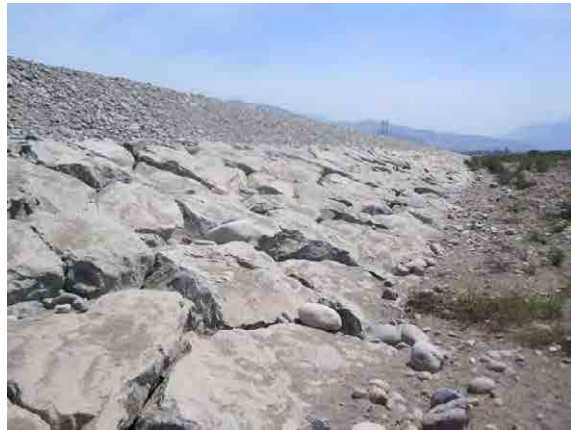
Figure 3.4 Dike and Revetment Works by Boulders in the Upstream in Pisco River
