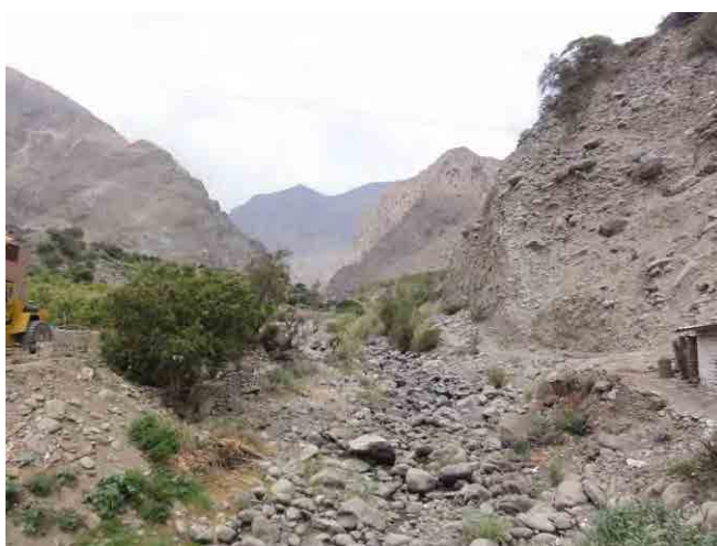
Figure 3.1.8-12 Andesitic and basaltic soil collapsed
