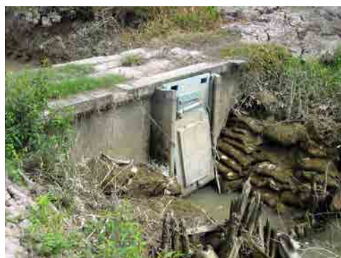
Tertiary canal gate
