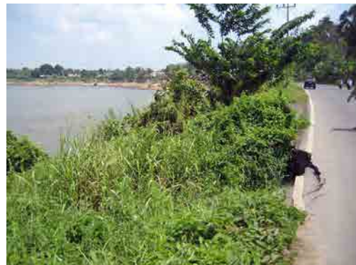
Damage of national road pavement due to Musi mainstream river bank erosion (Kec. Lais)
