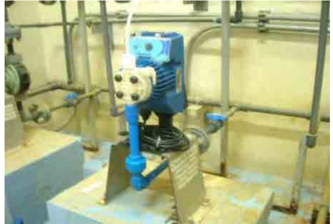
After rehabilitation: Post chlorination pump Pump is replaced and post chlorination can be done.
