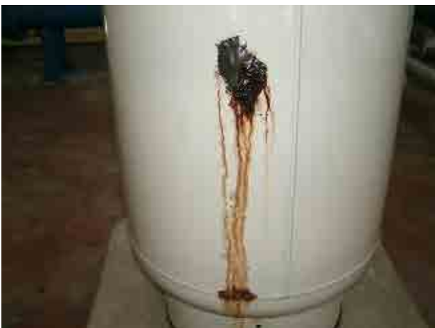
Before rehabilitation Pressure tank: The trace of leakage is found. It needs to be replaced.
