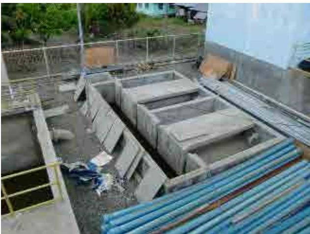
Before rehabilitation Sludge drying bed: Installation of bed sand is required due to accommodate the change in Philippines effluent standard.
