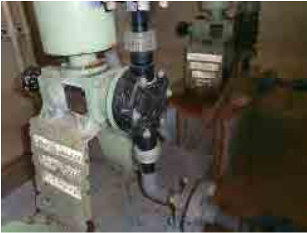
Before rehabilitation Post chlorination, injection pump: Not in use due to a breakdown.
