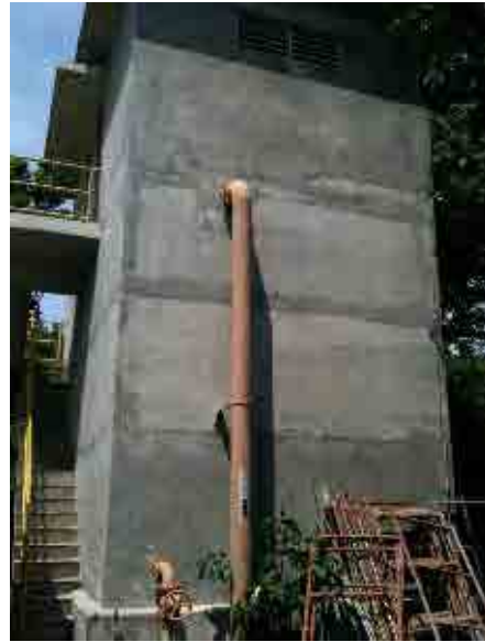
After rehabilitation Aeration tower: Removal of paint is completed and appearance became better.
