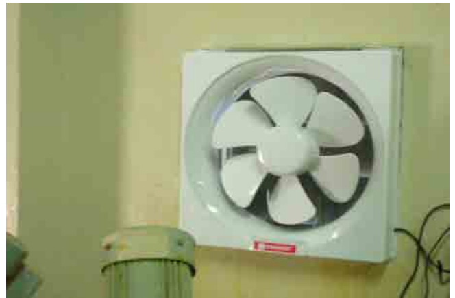
After rehabilitation: Chlorination room: Fan is replaced and the room is ventilated properly.
