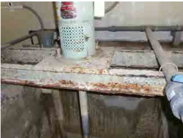
Before rehabilitation Chlorination agitator support: It was covered by rust of the corrosion.
