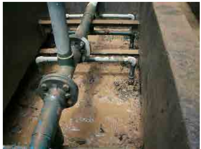
After rehabilitation Rapid sand filter Surface wash pipes were replaced to PVC and the surface became able to be washed properly.
