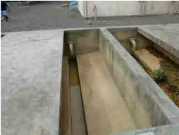
Before rehabilitation Sludge drying bed: Installation of bed sand is required due to accommodate the change in Philippines effluent standard..
