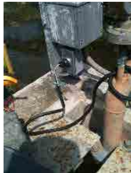
After rehabilitation Drainage basin: Outside consent for the single phase supply is installed, and the maintenance became easier.
