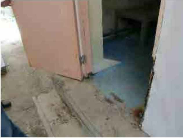
Before rehabilitation Chlorination room: The entrance door and its frame are corroded.
