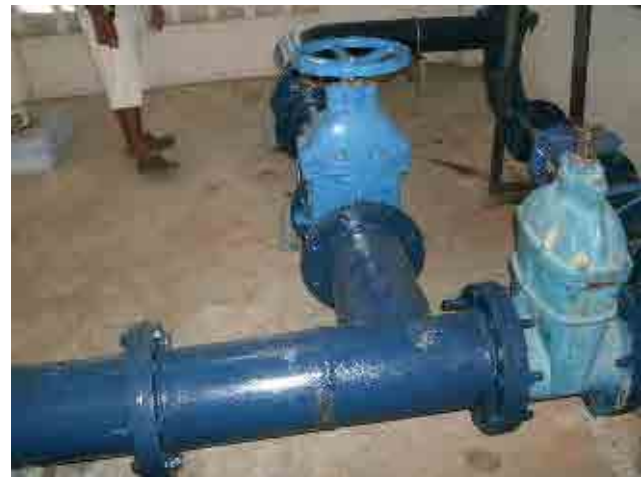
After rehabilitation Transmission pipes were installed and flow meter was replaced, so maintenance became easier.
