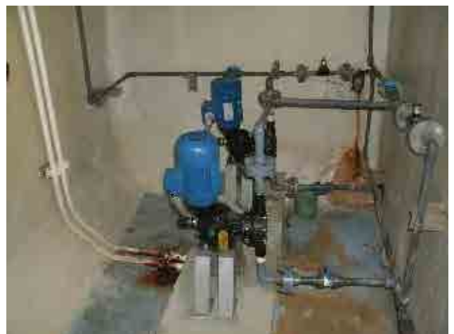
After rehabilitation Intermediate chlorination, injection pump: Pump is renewed and valve is installed to each injection pipe and it enabled equal injection to each pipe.
