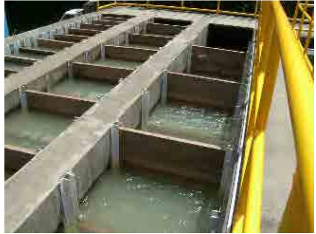
After Rehabilitation Flocculator: flow velocity is increased by adjusting the vertical baffles.
