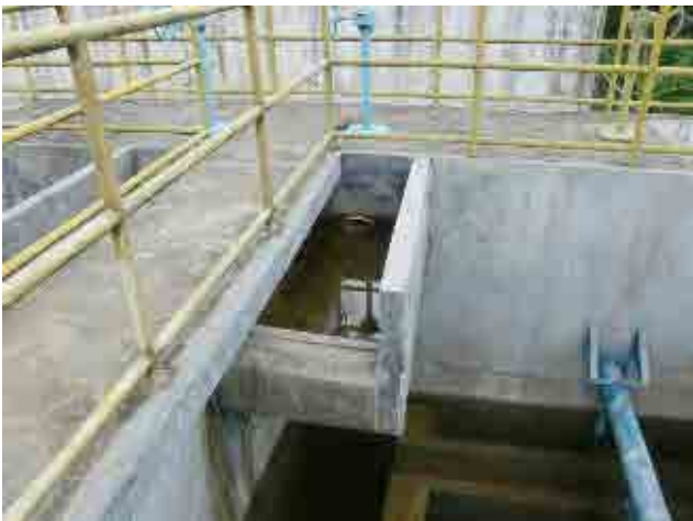
Before rehabilitation Rapid sand filter, inlet trough: Improvement is required to prevent flocs inflow to prevent the breakage.
