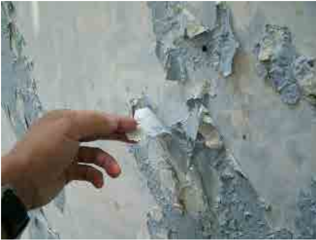
Before rehabilitation Aeration tower: Paint of exterior wall is peeled off. WD requested its removal.
