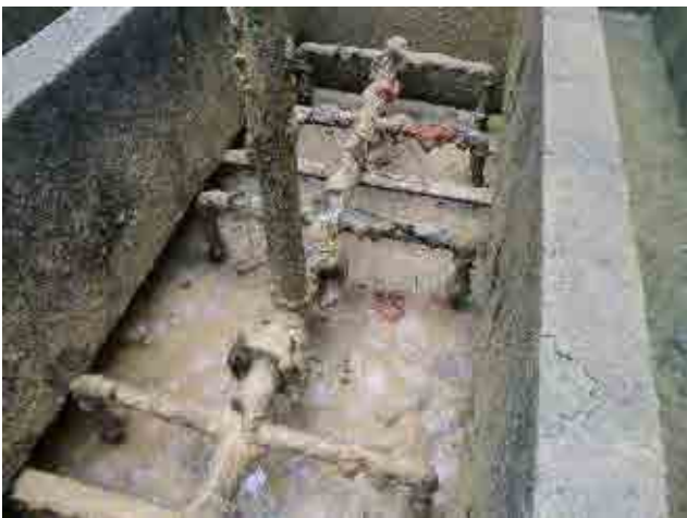
Before rehabilitation Rapid sand filter, surface-wash pipe: After drainage of water from the filter basin, settled flocs and sludge adhere to the surface-wash pipes.
