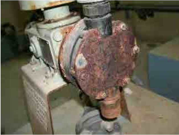
Before rehabilitation Post chlorination pump: Diaphragm part is malfunction due to corrosion. Post chlorination is missing.
