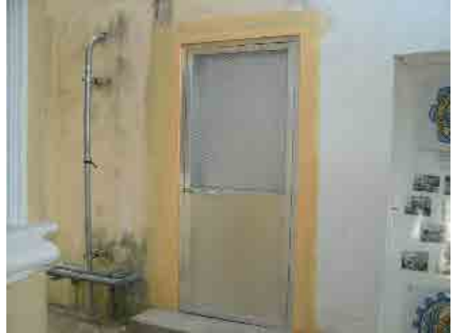
After rehabilitation: Door of chlorination facility: Replaced to aluminum double door and it will not be corroded.
