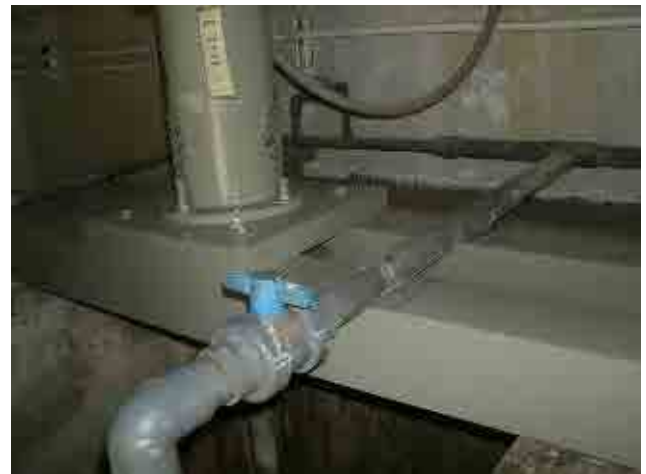
After rehabilitation Chlorination agitator support It was changed to wooden support, and durability is increased
