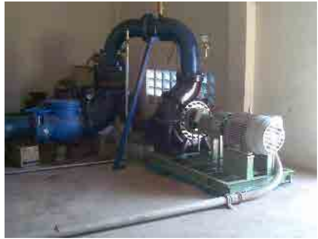
After rehabilitation Backwash pump Anti-corrosion pump is installed and backwash is done properly.
