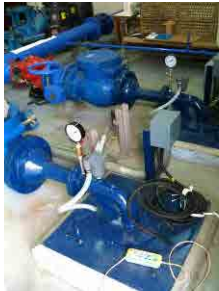
After rehabilitation: Distribution pumps: Replaced to submerged pump and water is distributed properly.
