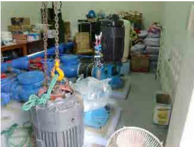
Before rehabilitation Distribution pumps: They are not in use due to a breakdown. Pump No.1 is not in use because of the broken shaft. Pump No.2 has a problem with over-current; the motor has no problem, thus the pump could be defective.
