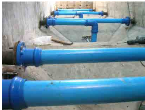
After rehabilitation Sedimentation basin: Corroded parts were replaced to PVC so as to drain properly and eliminate the risk of corrosion.
