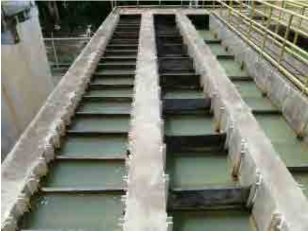
Before rehabilitation Hydraulic Flocculator: Adjustment of vertical baffles is required.
