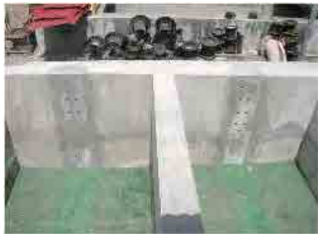
After rehabilitation Sludge Drying bed: Gravel and sand are filled and re-graded. Tank volume is appropriate for the drying purpose.
