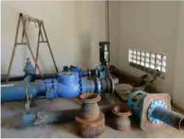
Before rehabilitation Backwash pump: It has been removed since Oct 2009 because of a breakdown.
