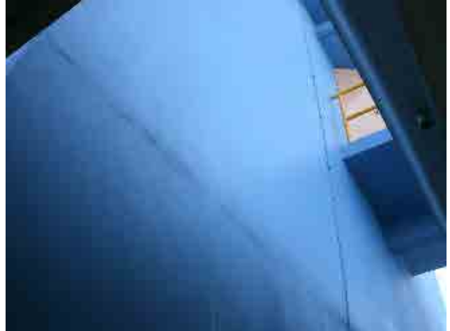
After rehabilitation: Aeration tower: Leakage part was repaired and each facilities were painted.
