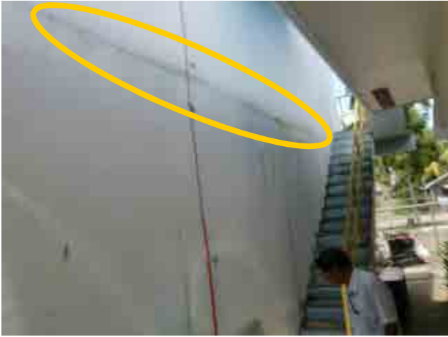
Before rehabilitation Aeration Tower: Leakage from the concrete joint.
