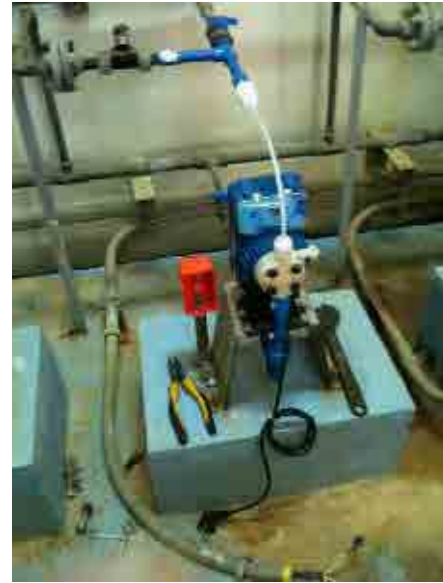
After rehabilitation Post Chlorination injection pump Pump is renewed so post chlorination can be done.
