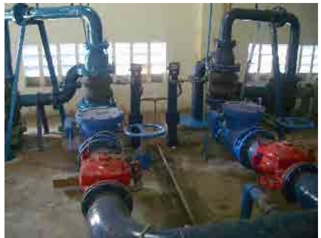
After rehabilitation Transmission and distribution pump The pumps were replaced to the anti-corrosion ones and the concern of rusting was resolved.
