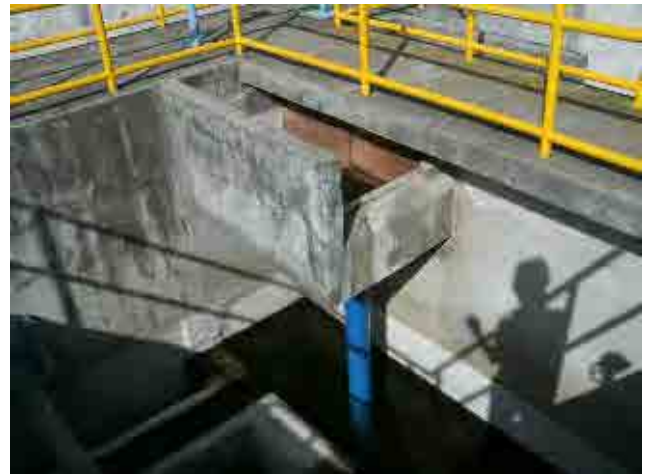
After rehabilitation Rapid sand filter: Inlet pipe was installed to prevent floc breakage
