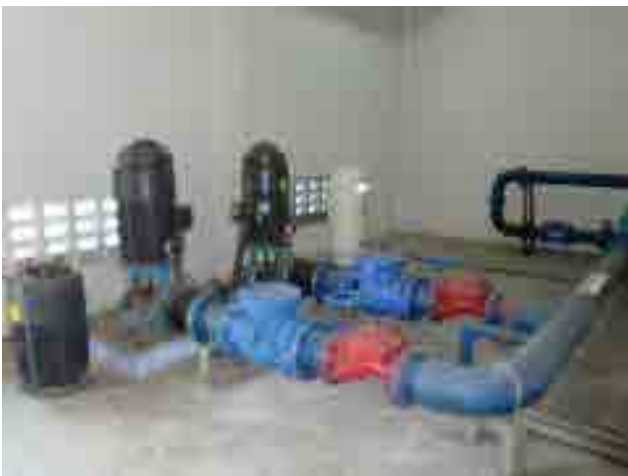
Before rehabilitation Transmission and distribution pump Pumps were wearing out with corrosion. There is the risk of sudden interruption.
