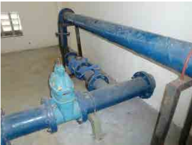
Before rehabilitation Transmission pipe: A bypass line is connected from another water source to dilute the saline water in the reservoir.
