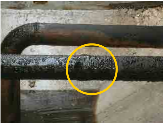
Before rehabilitation Sedimentation basin: Hole on the sludge drain pipe has been repaired with rubber sheet.
