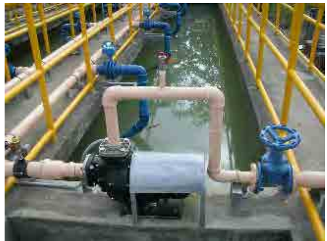
After rehabilitation Sedimentation basin, sludge drain pipes: Sludge pump and distribution pipes are installed, and operated properly
