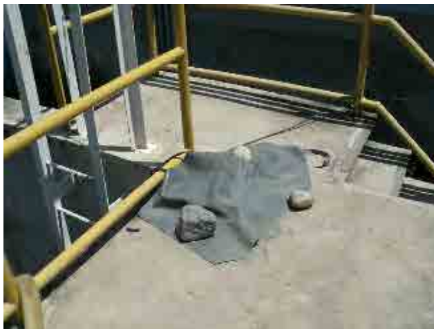
Before rehabilitation Drainage basin: The single phase socket is covered by a sheet for insulation.
