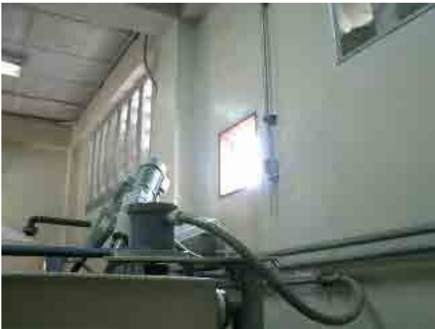
Before rehabilitation Chlorination room: Ventilation fan has been removed due to breakdown.
