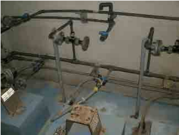
Before rehabilitation Post chlorination pump: It has been removed due to breakdown.
