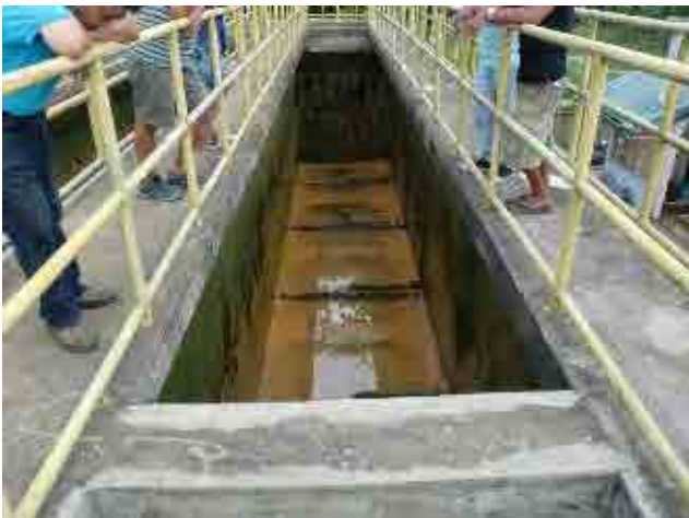
Before rehabilitation Sedimentation basin, sludge drain pipes: All pipes are corroded by high salinity of the raw water.
