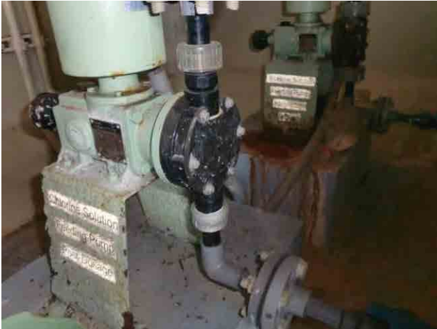
Post chlorination, injection pump: Not in use due to the breakdown.
