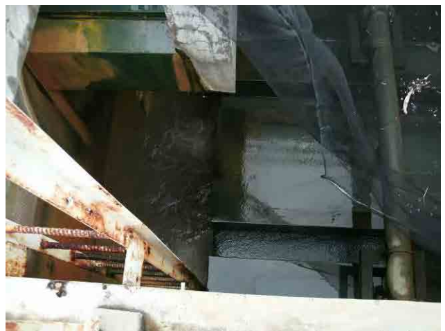
Rapid sand filter: After the back wash.
