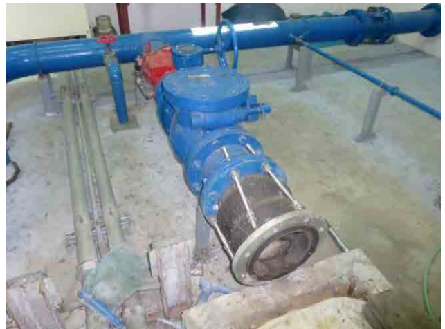
Transmission pump: No.2 has removed due to the mechanical failures.
