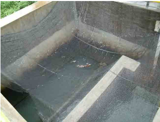
Rapid sand filter: Filter basins are covered by the net to prevent the leaves dropping in.
