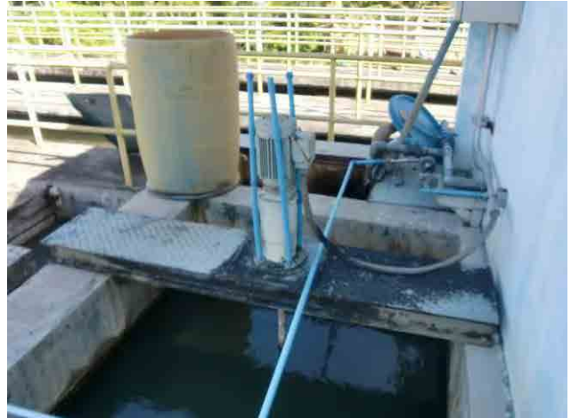
Rapid mixer: Not in use due to breakdown. It was covered not to hit rain and it was decomposed and greased once.
