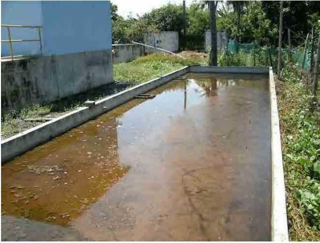
Sludge Storage basin: It takes about 3-4 weeks for drying sludge by natural evaporation in the sludge storage basin.
