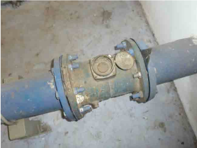
Flow meter for surface-wash pipe: Flow meter has been removed.
