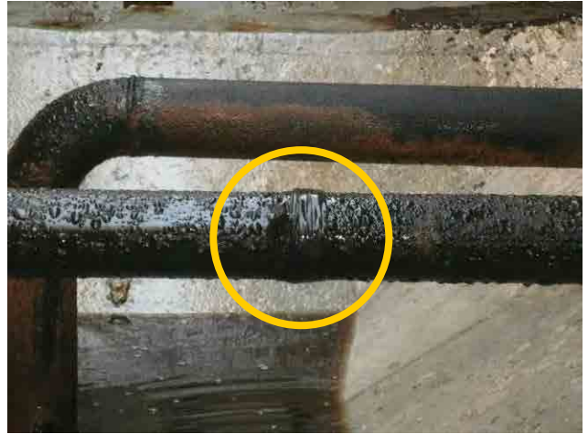
Sedimentation basin: Hole on the sludge drain pipe has been repaired with rubber sheet.
