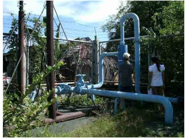
No.7 Well: Quantity of water intake is 10.5l/s which is less than planned value, 28l/s.
