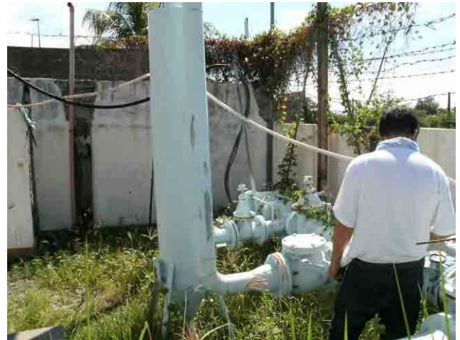
No.6 well: Quantity of water intake is 24.4l/s which is close to planned value, 28l/s.
