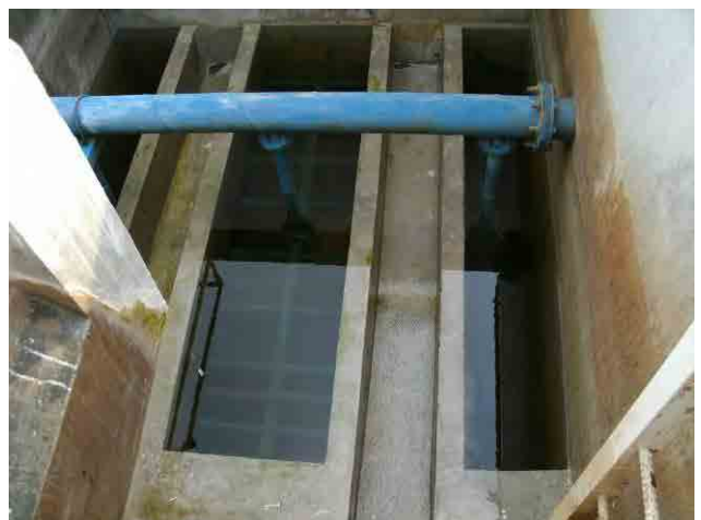
Rapid sand filter: After backwash the water is relatively clear.
