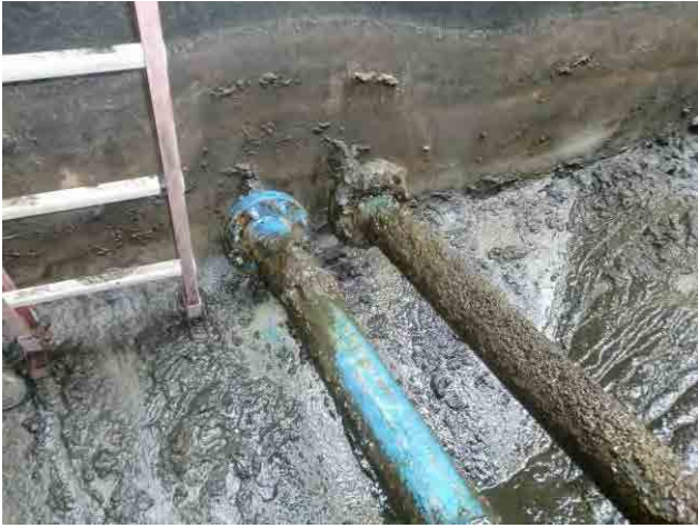
Sedimentation basin, sludge drain pipes: Pipes are not corroded; however, the sludge is attached on the pipes.
