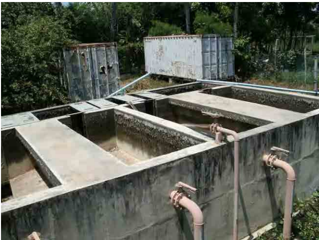
Sludge drying bed: Bed sand has been removed due to clogging after being used for five times.
