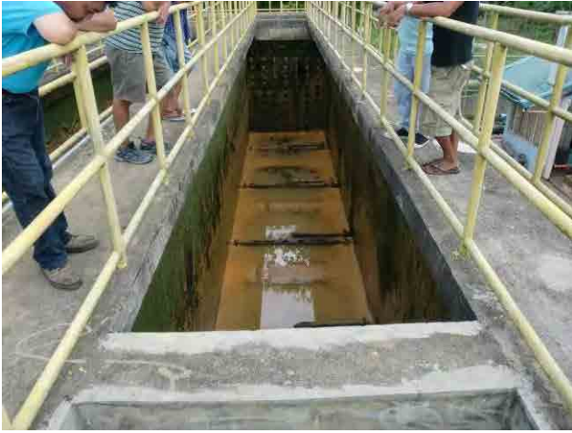
Sedimentation basin, sludge drain pipes: All pipes are corroded by high salinity of the raw water.
