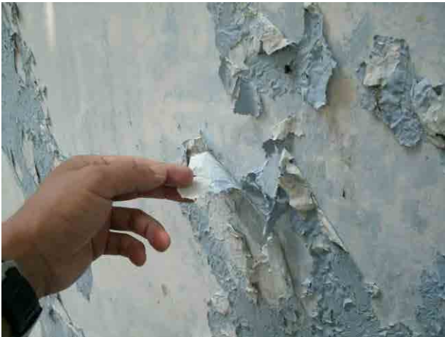
Aeration tower: Paint of exterior wall is peeling off. WD requested to remove all.
