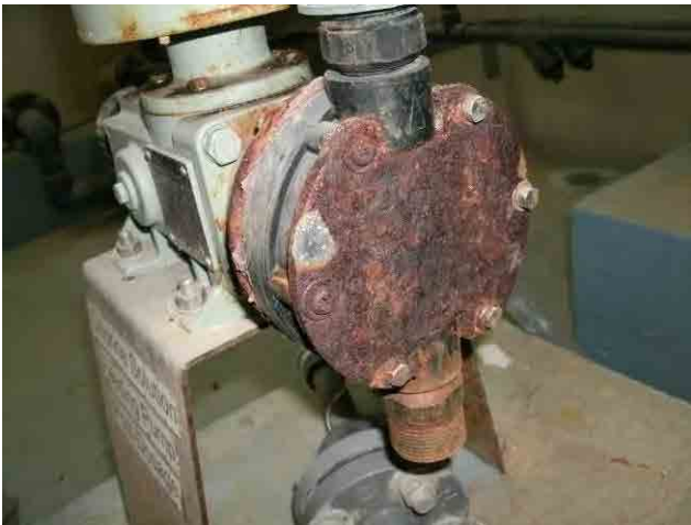
Post chlorination pump: Diaphragm part is malfunction due to corrosion. Post chlorination is missing.
