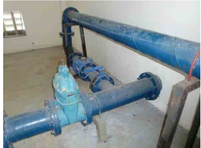
Transmission pipe: A bypass line is connected from another water source to dilute the saline water in the reservoir.
