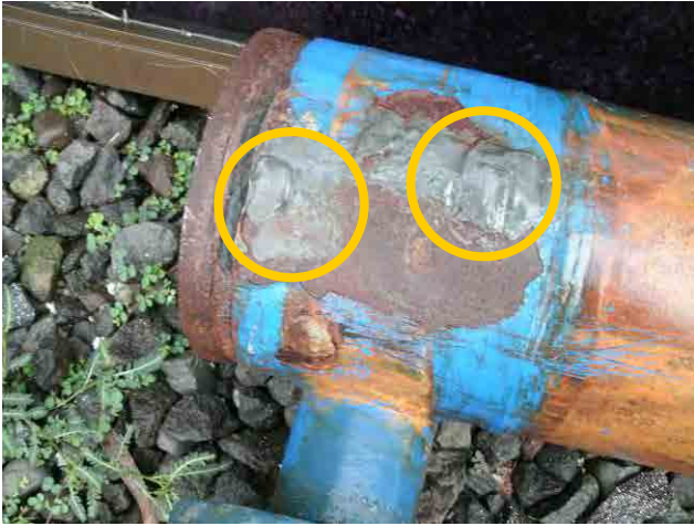
Sand separator: Holes have been filled with pate.
