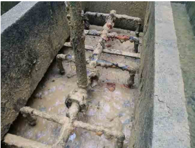
Rapid sand filter, surface-wash pipe: After drainage of water from the filter basin, settled flocs and sludge adhere to the surface-wash pipes.
