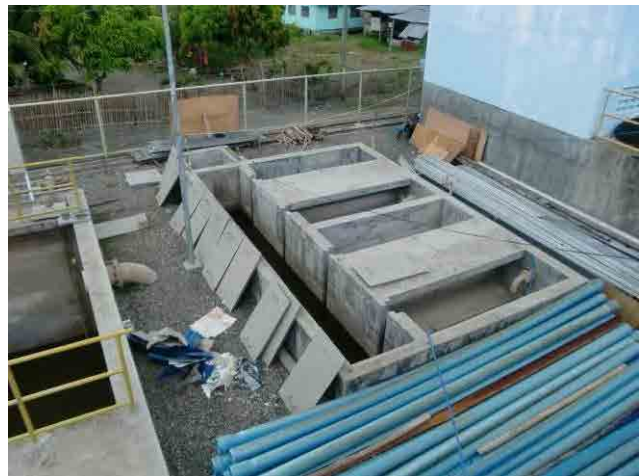
Sludge drying bed: Installation of bed sand is required due to accommodate the change in Philippines effluent standard..
