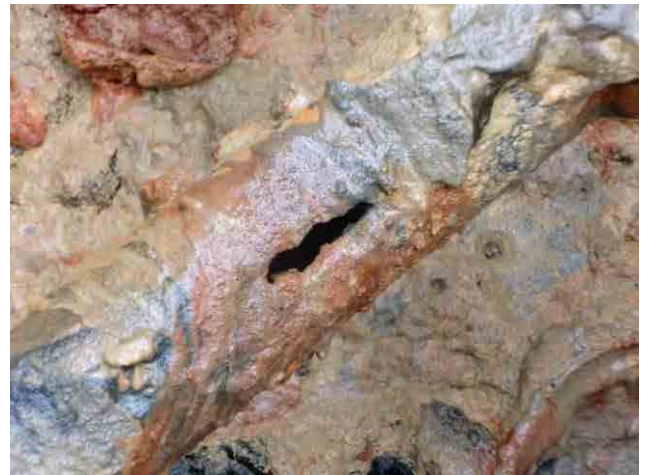
Rapid sand filter, surface-wash pipe: Contact with saline flocs caused corrosion, making holes on the surface-wash pipe.
