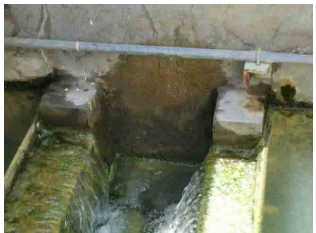
Intermediate chlorination, injection pipe: Chlorine injection at 4 injection points is not even.
