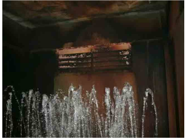
Aeration tower: Water pressure decreased so the jet does not reach to the ceiling. DO in the water is sufficient.
