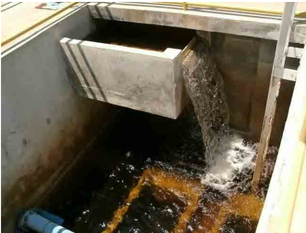
Rapid sand filter: Inlet structure needs to be modified to avoid small flocs breakdown.
