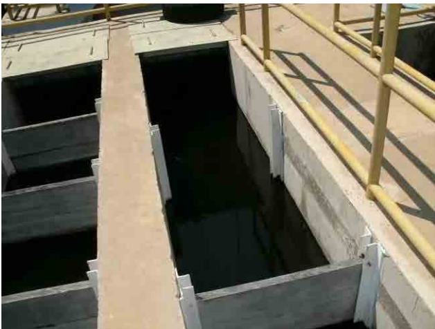
Flocculator: Last two lines of baffle plates were removed for cleaning.
