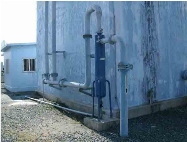
Sand separator: Sand raise is observed.
