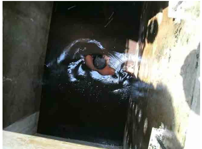
Sedimentation basin: Sludge is accumulated at the end of the basin.
