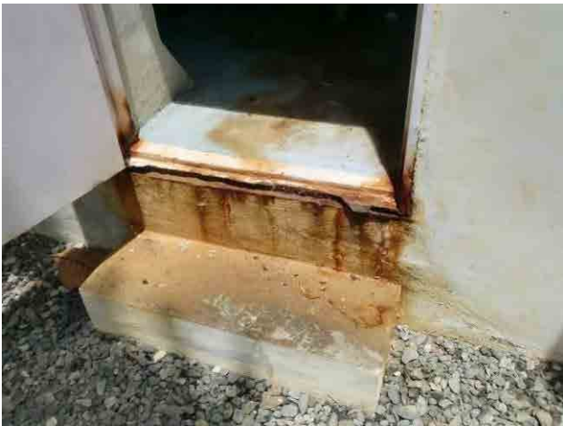
Chlorination room: The entrance door and its frame are corroded and decayed.
