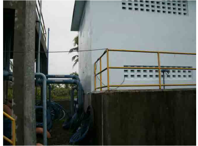
Chlorination pump: Single phase power is supplied by using the extension electric cord.
