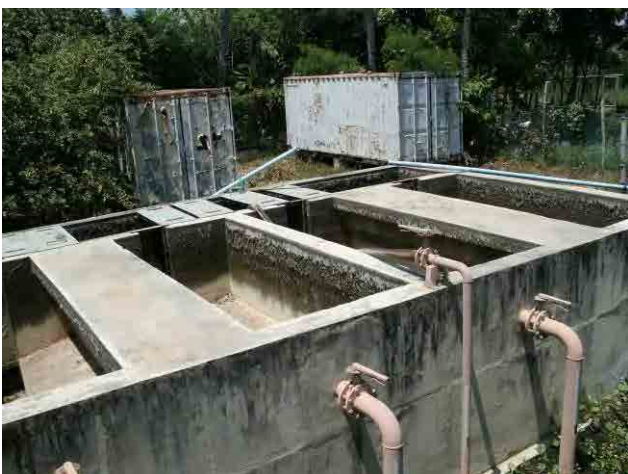
Sludge drying bed: Bed sand has been removed due to causing clog after using five times.
