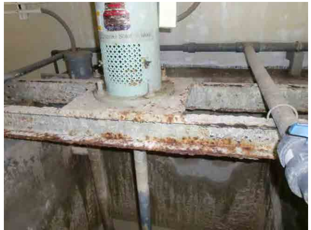
Chlorination agitator support: Covered by rust of corrosion.
