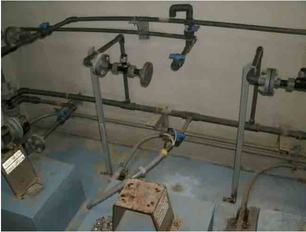
Post chlorination pump: It has been removed due to breakdown.
