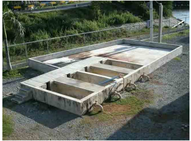
Sludge Drying bed: An additional sludge storage basin was constructed by WD for receiving the excess sludge.
