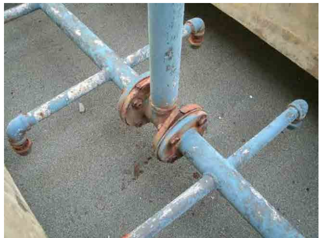
Rapid sand filter: Surface wash pipe needs to be repaired due to rust.
