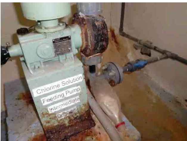
Pre/Intermediate chlorination, injection pump: Leakage from diaphragm of the pump.
