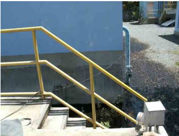
Drainage basin: The single phase power is provided from the distribution pump room using an extension cord.
