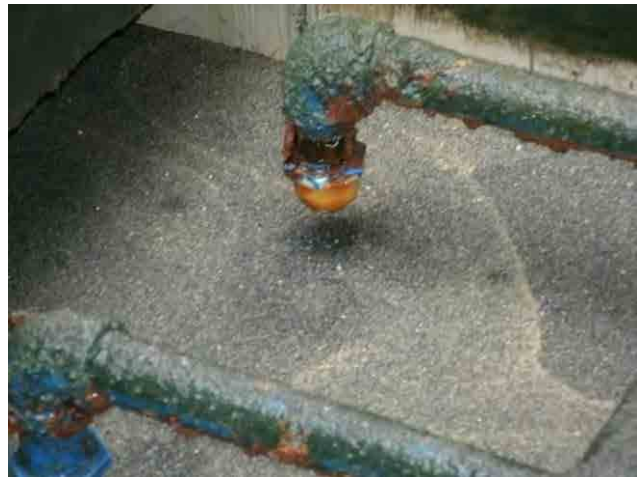
Rapid sand filter: Surface-wash pipes are corroded thus need to be repaired.
