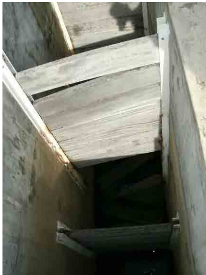
Flocculator: Some baffle plates fell off due to breakage of holding bolts caused by corrosion.
