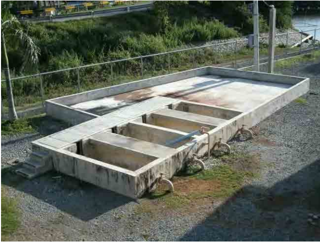
Sludge Drying bed: An additional sludge storage basin was constructed by WD to receive the excess sludge.
