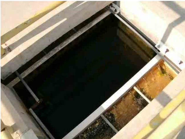
Sedimentation basin: Flocs are carried over from the effluent trough.
