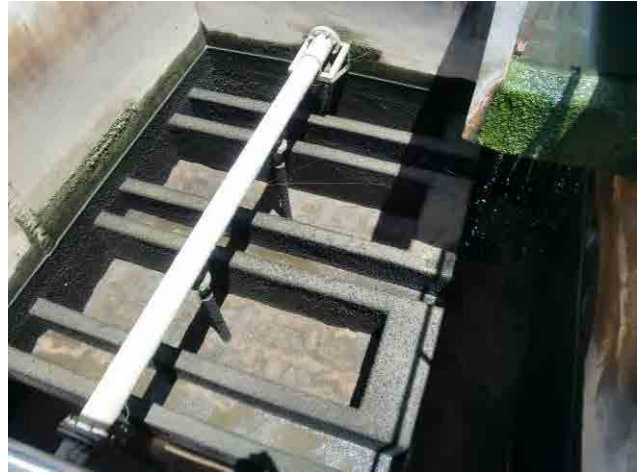
Rapid sand filter: Filter sand is put more than requires, it must be removed.
