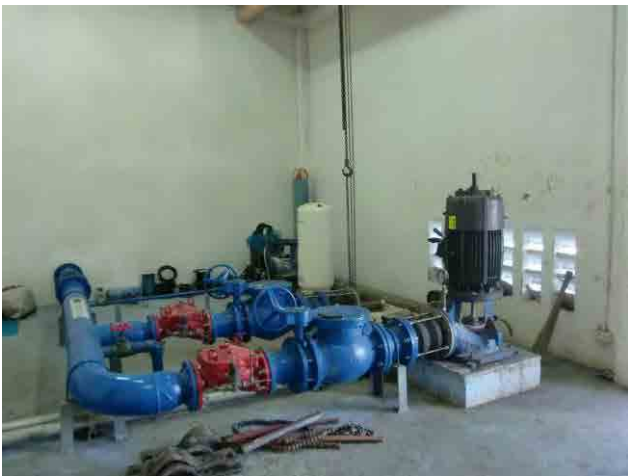
Transmission pump: No.2 pump is not in use due to shaft broken. The moter is no problem. Currently No.1 and surface-wash pump are operated alternatively.
