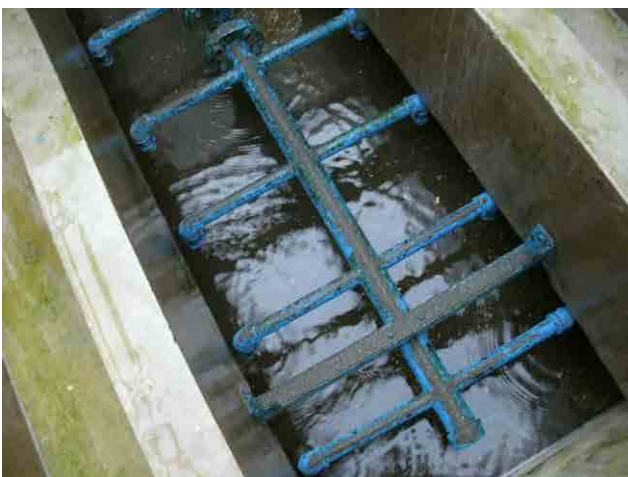
Rapid sand filter: Backwashing of the filter sand
