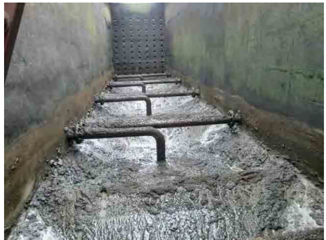
Sedimentation basin: Sludge is black, it might be manganese.
