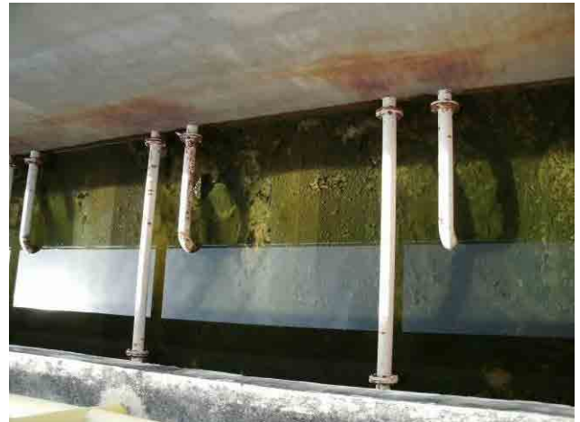
Sedimentation basin: Pipes need waterproof painting due to rust.
