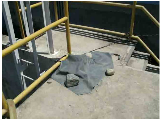
Drainage basin: The single phase socket is covered by a sheet for insulation.
