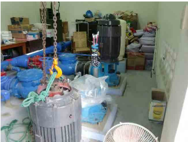
Distribution pumps: Not in use due to breakdown. Pump No.1 has a broken shaft. Pump No.2 has a problem with over-current; the motor has no problem, thus a problem in the pump is presumed.
