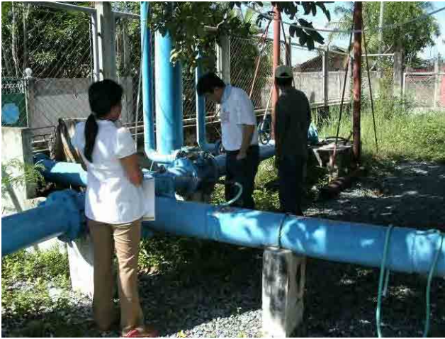
No.4 Well: Quantity of water intake is 11l/s, which is less than planned value, 28l/s.
