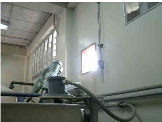
Chlorination room: Ventilation fan has been removed due to breakdown.
