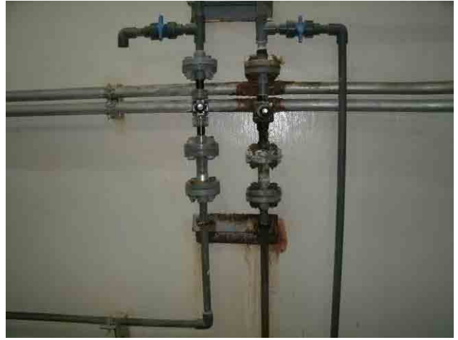
Pre/Intermediate chlorination pipe: Some parts are corroded.
