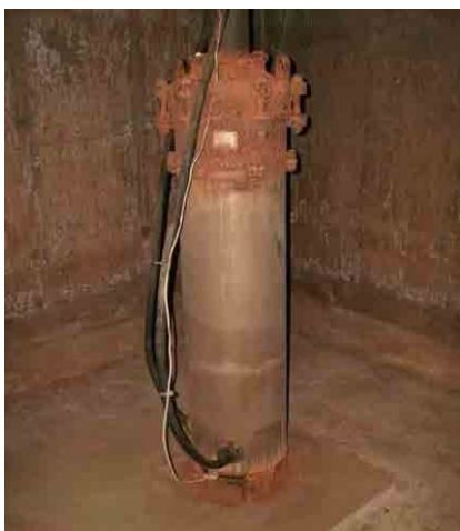
Distribution pump: Rusting but no problem for operation.
