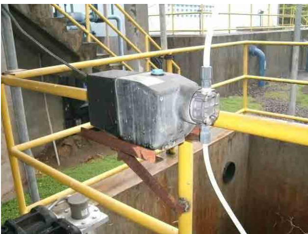
Intermediate Chlorination pump: installed by the WD
