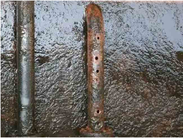
Sedimentation basin: Sludge drain pipe has holes due to corrosion.
