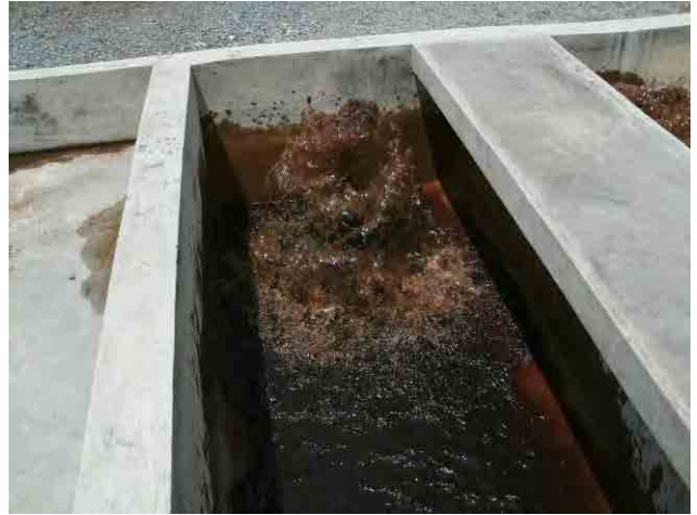
Sludge Drying bed: Drained sludge is being discharged into the drying bed.
