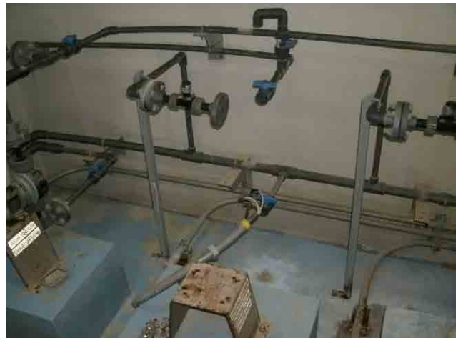
Post chlorination pump: It has been removed due to a breakdown.
