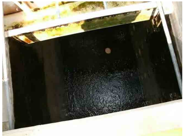
Sedimentation basin: Due to insufficient settlement of flocs, sludge is accumulated at the end of the basin.
