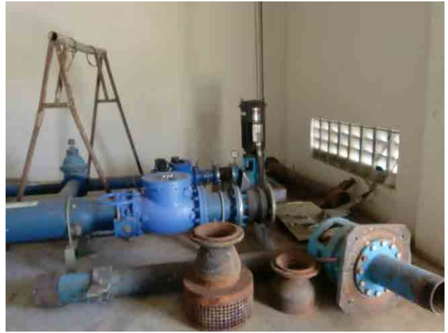
Backwash pump: It has been removed since Oct 2009 because of mechanical failures.
