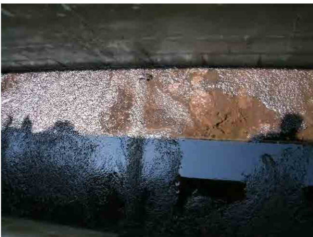
Sedimentation basin: A large amount of blown sludge is accumulated.
