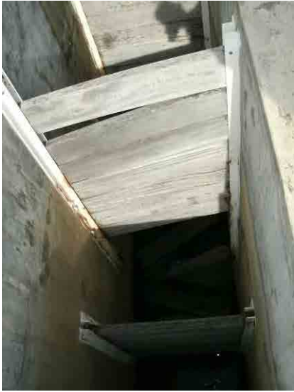
Flocculator: Some baffle plates fell off due to breakage of holding bolts caused by corrosion.
