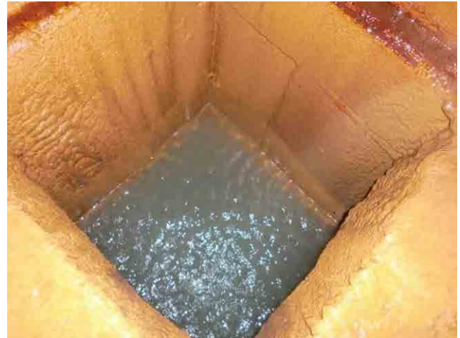
Aeration tower: There are no steps for existing manholes. New manholes will be opened for effective maintenance.
