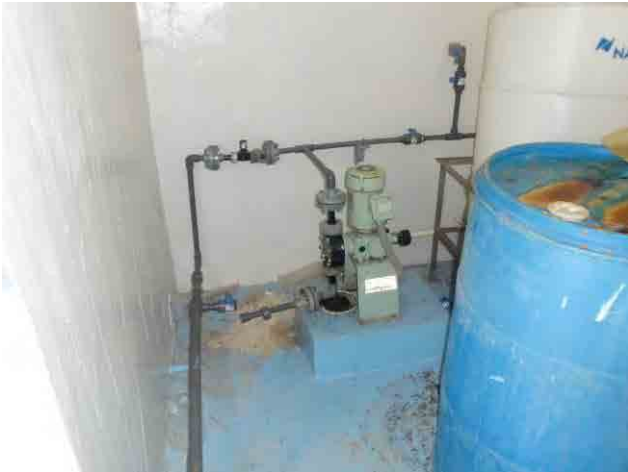
Chemical feeding pump: broken down and not being used.
