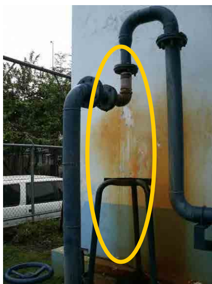
Sand separator: It was changed two times and finally removed because of holes.
