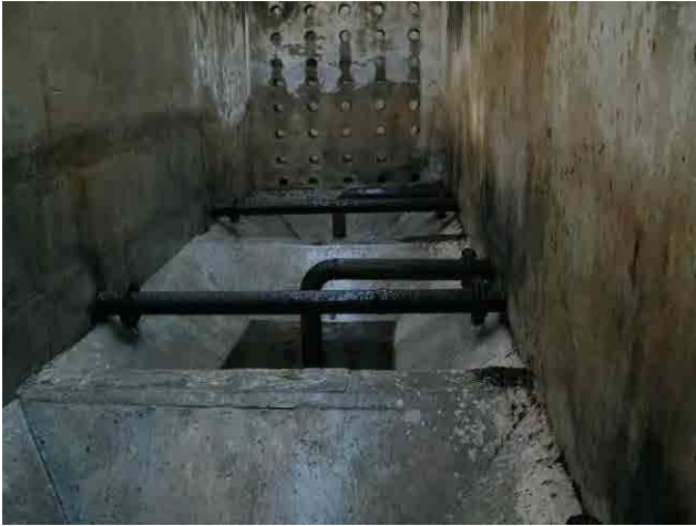
Sedimentation basin: Paint of sludge drain pipe peels off and some pipes are corroded.
