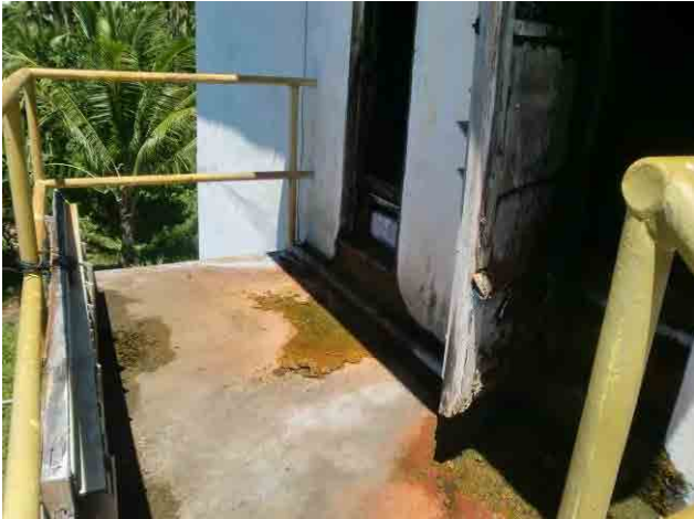
Aeration tower: The doors are decrepit; one of doors is already removed.
