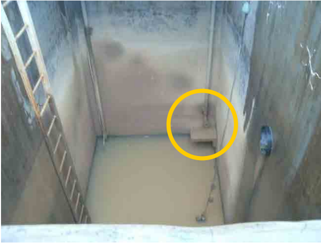
Drainage basin: Recycle pump has been removed due to breakdown.
