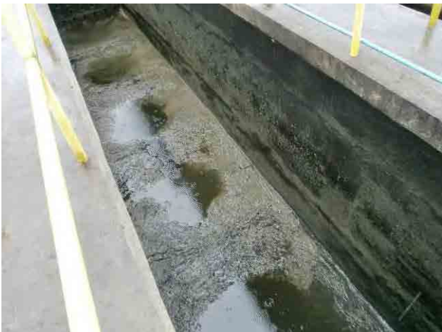
Sedimentation basin: Sludge is removed only three times since the operation started. Therefore, the sludge is accumulated considerably.
