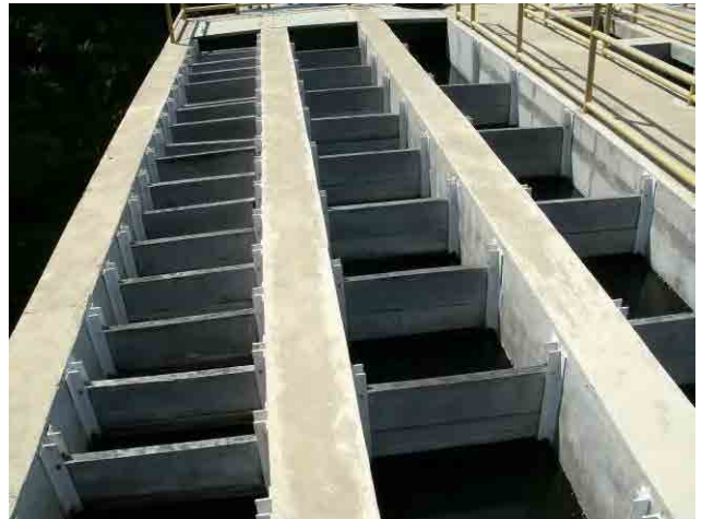
Flocculator: Some baffle plates fell off due to breakage of holding bolts by corrosion.
