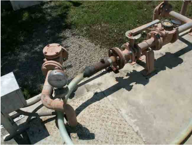
Drainage basin: Recycle pump has been replaced with a single phase pump and connected to existing pipe by WD.
