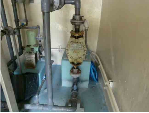
Intermediate chlorination, injection pump: Although it often stops due to mechanical failures, it is decomposed and fixed and so it can be used somehow.
