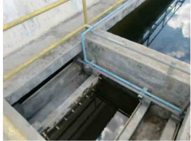
Intermediate chlorination, injection pipe: Chlorine injection at 4 injection points is not even.
