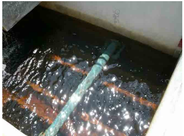
Rapid sand filter: Colored particles are not removed in the sedimentation basin, thus the influent water is colored.
