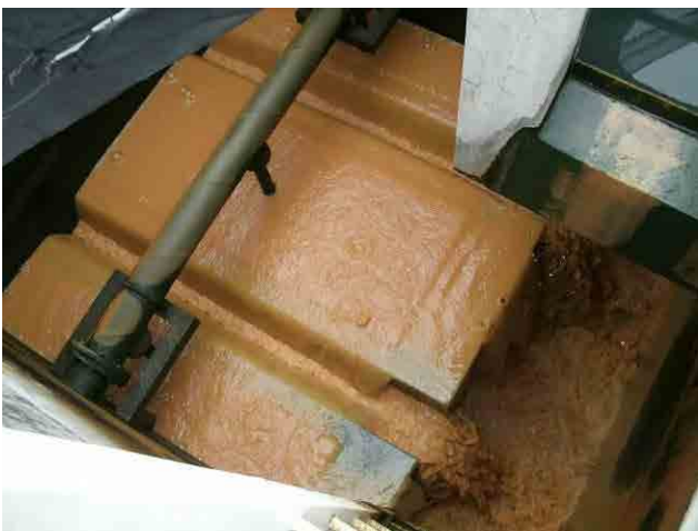
Rapid sand filter: Under back washing.
