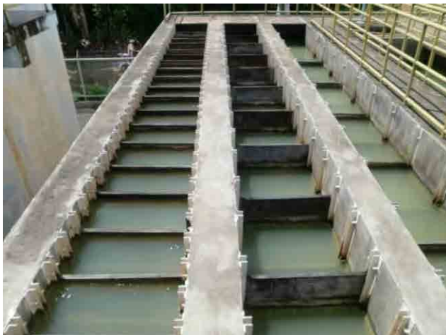
Hydraulic Flocculator: Adjustment of vertical baffles is required.
