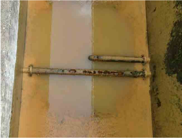
Sedimentation basin, sludge drain pipes: Corrosion makes holes on the pipe.
