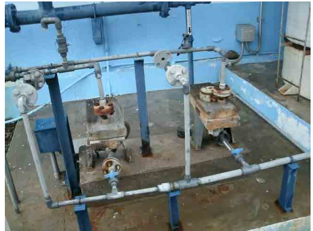
Chlorination pump: Pumps were removed because of Corrosion.
