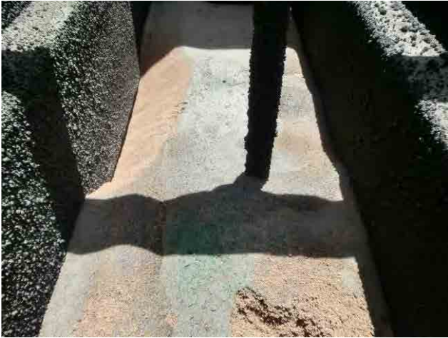
Rapid sand filter: A sand layer thickness is 60cm by the plan, but currently 90cm; thus the surface-wash pipes are covered and filtration area has decreased due to no space between sand and trough.
