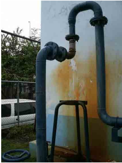
Sand separator: It was changed two times and finally removed because of holes.
