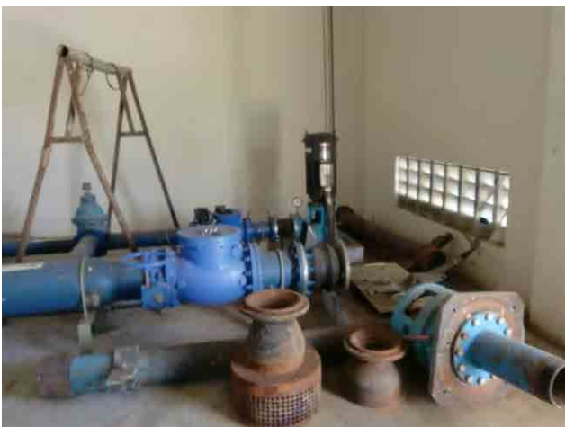
Backwash pump: It has been removed since Oct 2009 because of mechanical failures.
