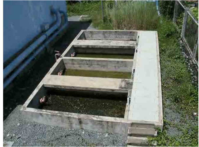
Sludge drying bed: Gravel has been filled but it is not used.
