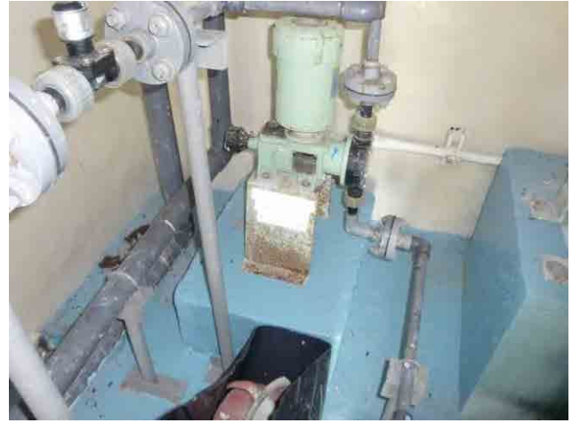
Post chlorination, injection pump: broken down; does not work when it is powered on.
