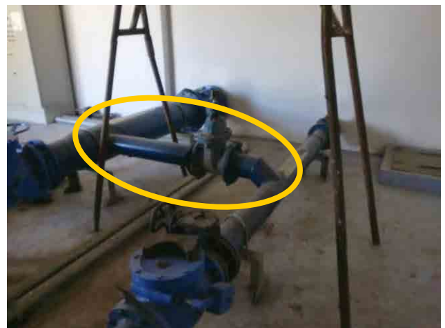
Backwash pipe: Bypass connection from the surface-wash pipe was installed as an emergency measure.
