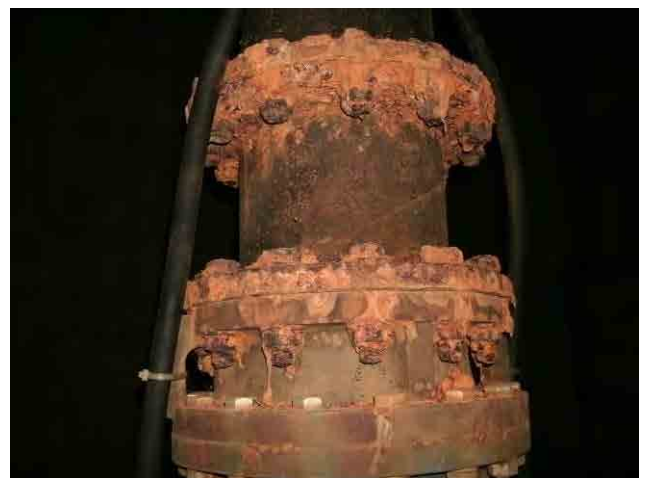
Back wash pump: Rusting but no problem for operation.
