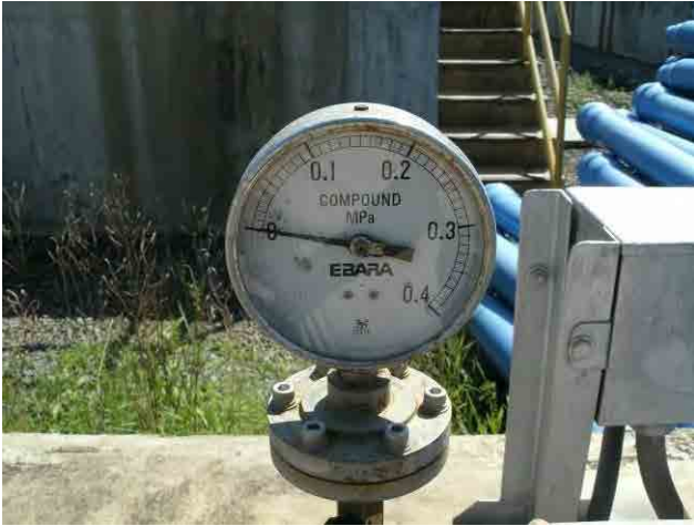
Pressure gauge for Recycle pump: Pressure gauge is broken.
