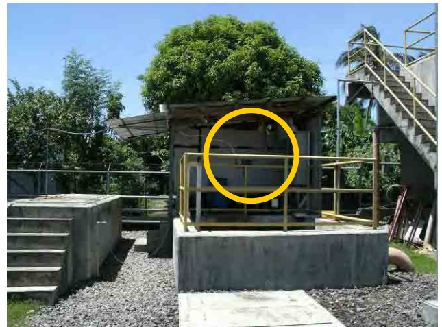
Intermediate Chlorination pump: installed by the WD
