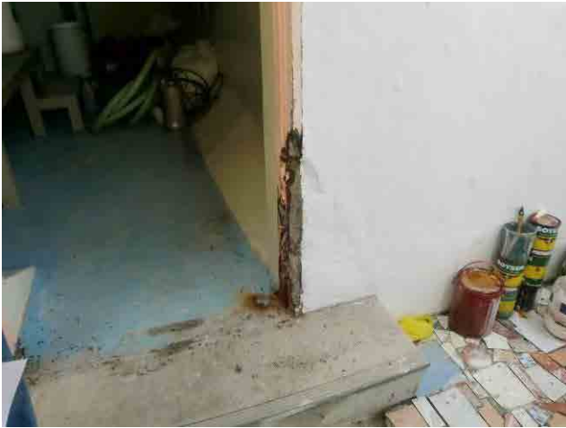
Chlorination room: The entrance door and its frame are corroded.
