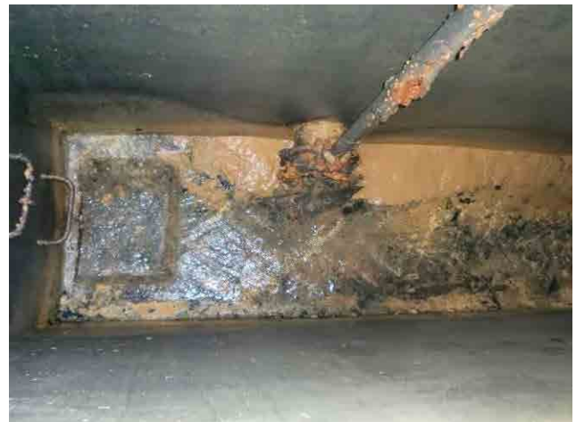
Sedimentation basin, inlet valve: Covered by lumps of rust due to corrosion.
