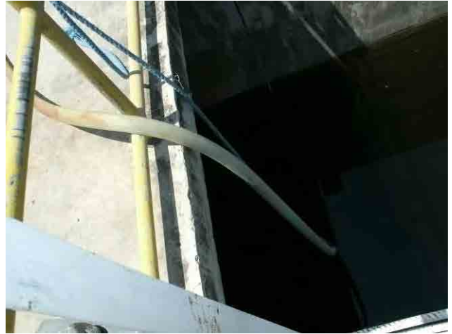
Drainage basin: The single phase pump installed by WD.
