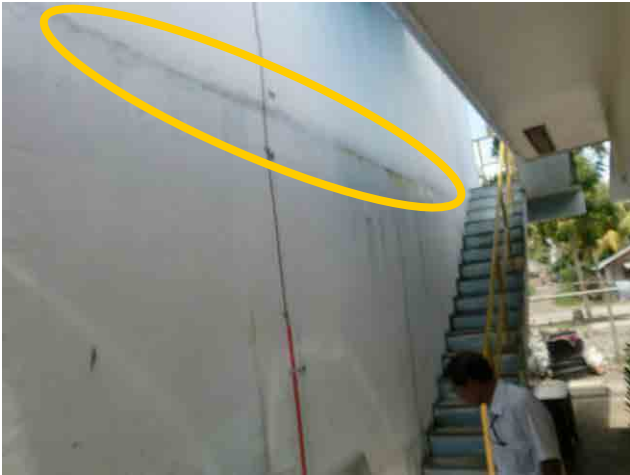
Aeration Tower: Leakage from the concrete joint.
