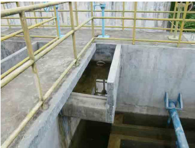
Rapid sand filter, inlet trough: Improvement is required to prevent the destruction of the floc.
