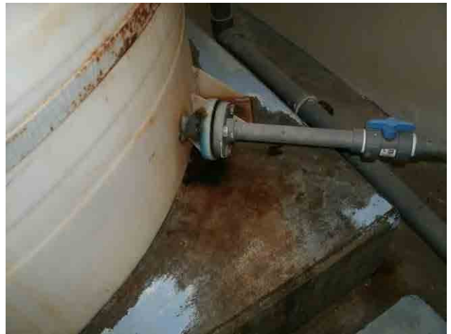
Chlorine tank: Leakage of chlorine solution at the pipe connection is observed.
