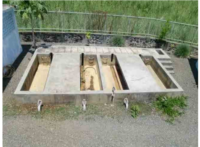
Sludge drying bed: Installation of bed sand is required due to accommodate the change in Philippines effluent standard..
