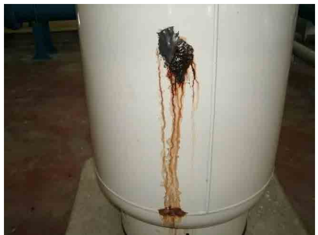
Pressure tank: The trace of leakage is found. It needs to be replaced.
