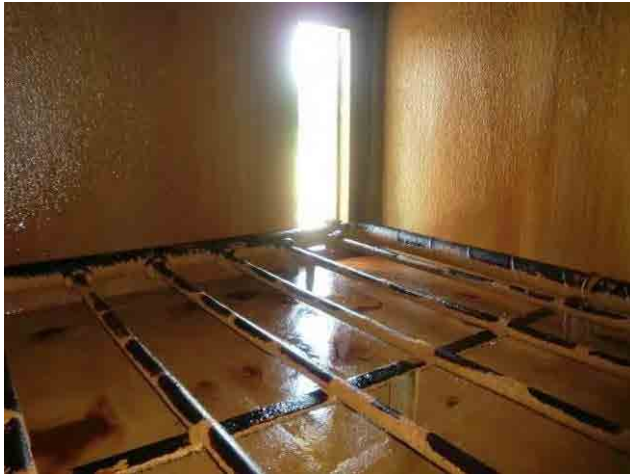
Aeration tower: Oxygen concentration is sufficient.
