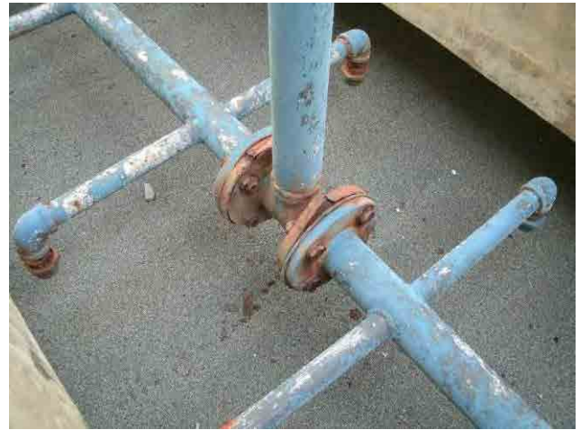
Rapid sand filter: Surface wash pipe needs to be repaired due to rust.
