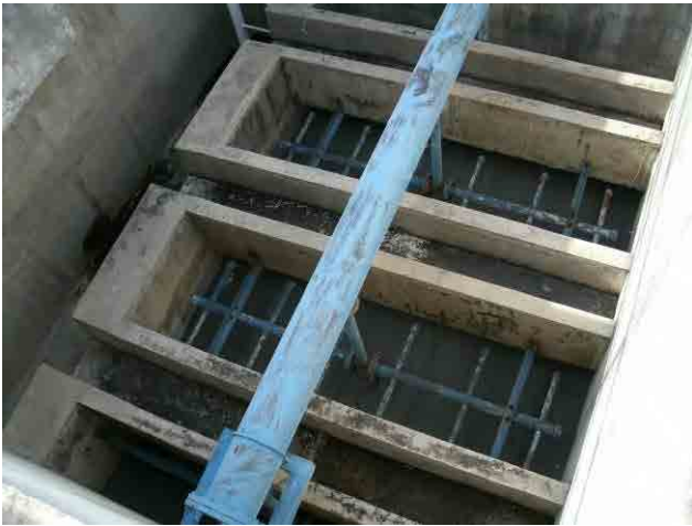
Rapid sand filter: Surface wash pipe needs to be repaired due to rust.
