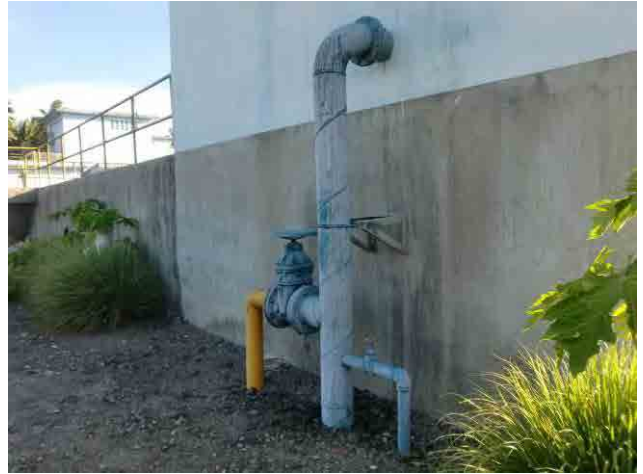
Rapid sand filter, surface-wash pipe: Currently the surface-wash pump is used as transmission pump, thus the surface-wash is not conducted now. This is the major factors that caused the mud ball.
