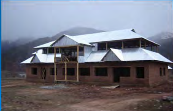
New office of Beekeeping Support Center, square 242 sq. m, built by people of the region, migrants families by the method of "Hashar"
