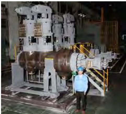
Photo 165-1 Main stop valve
