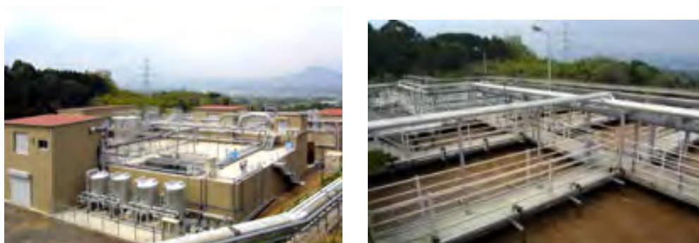
Photo 228-1 Wastewater treatment equipment
