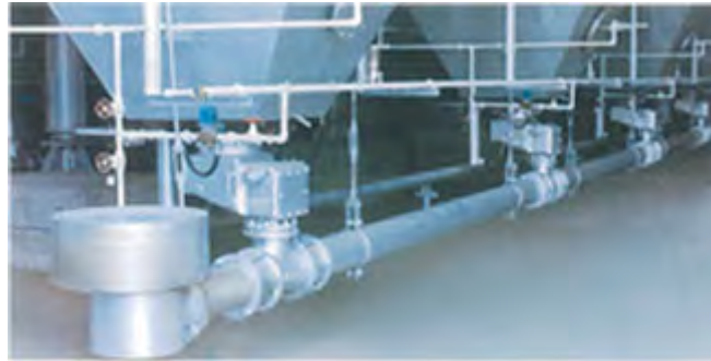
Photo 245-2 Fly ash disposal system (Vacuum transportation system)
