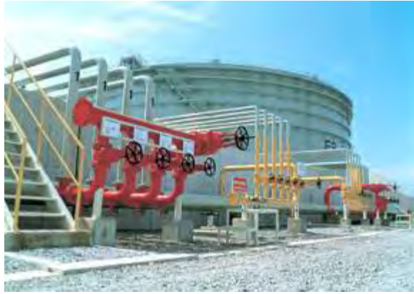
Photo 121-1 Foam fire extinguishing system
