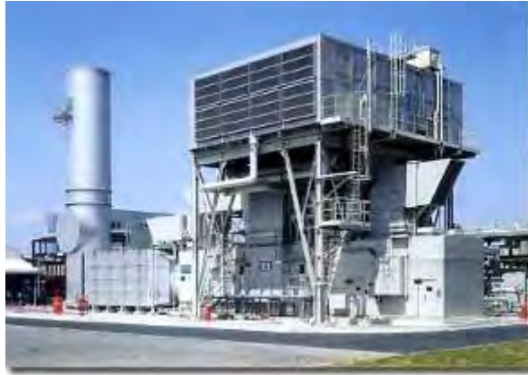
Photo 191-1 Air intake room
