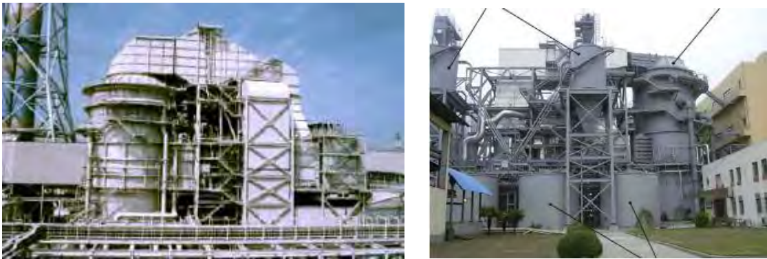
Photo 152-5 De-SO x equipment (Absorber)
