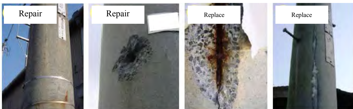
Figure 44 Example of cracks on concrete poles
